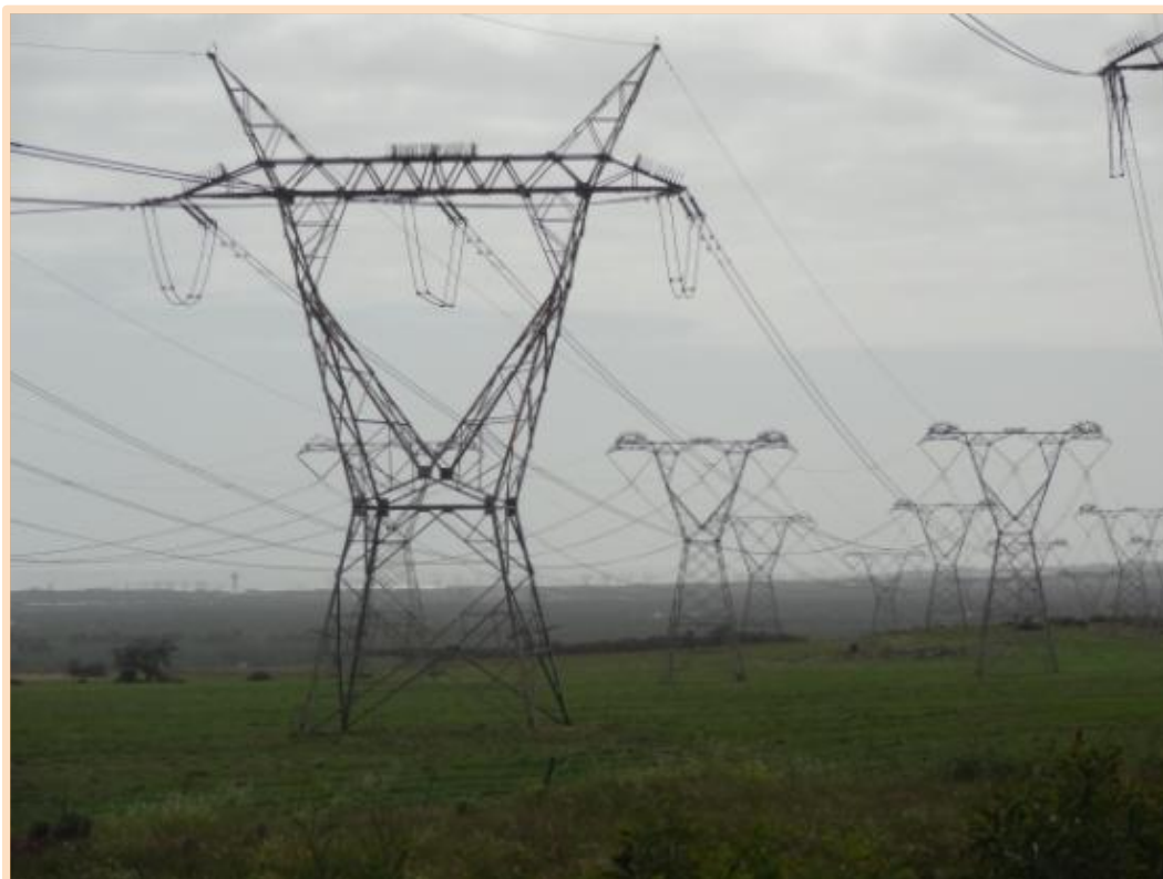
Plate 1: View of an example of self-supporting strain tower powerline.
