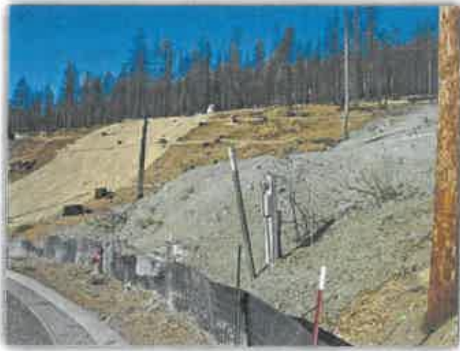
Figure 6 the use of a reinforced silt fence hold back the soil from washing into the road during construction
