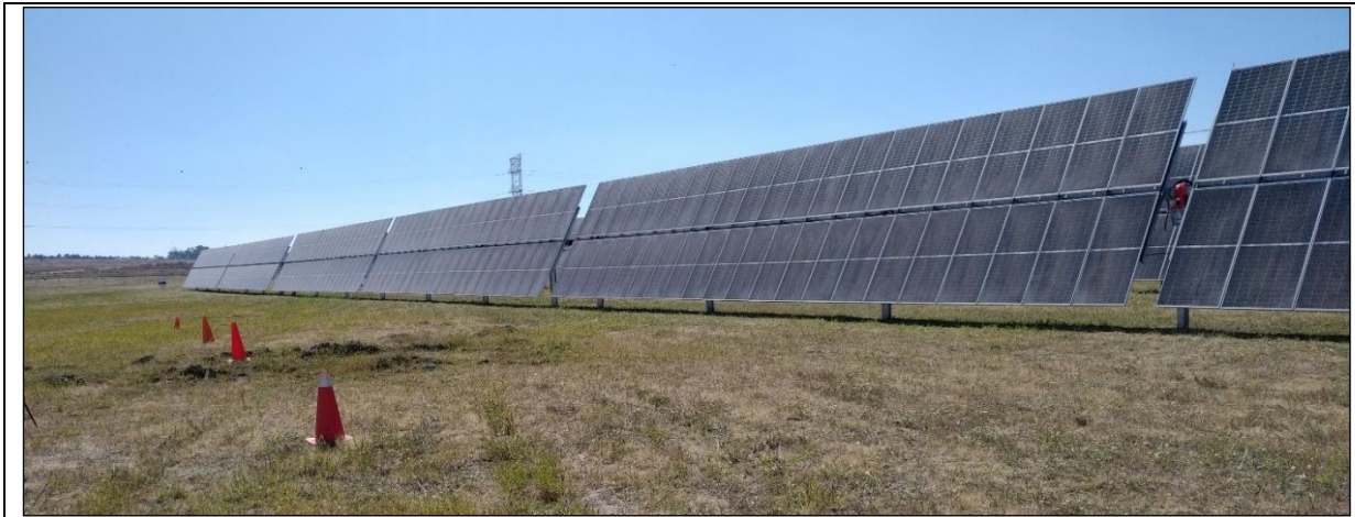
Plate 4-4: Frontal views of the PV arrays mounted on horizontal 1-axis tracker
