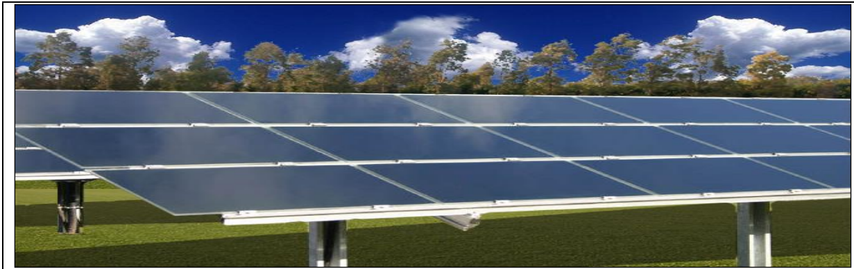
Plate 4-2: Frontal view of PV arrays mounted on fixed mounting systems
