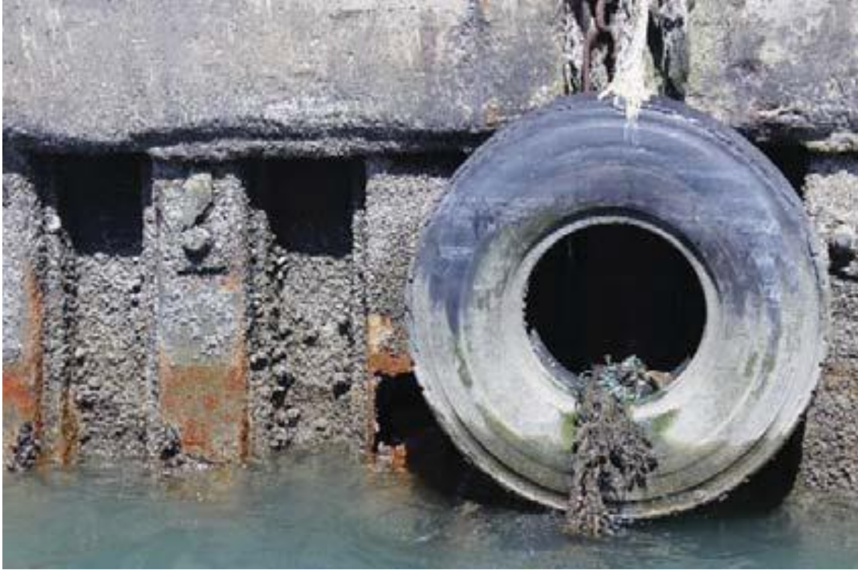
Figure 3: Close-up image indicating the extent of the sheet pile corrosion
