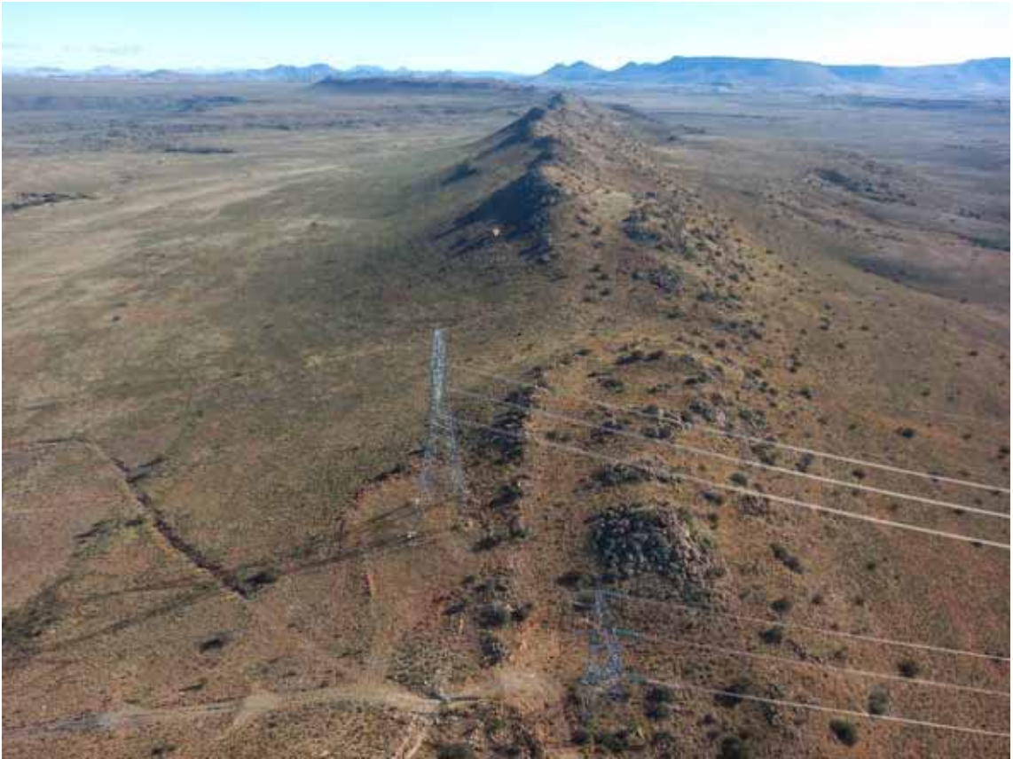
Existing gridline infrastructure on the eastern side of the Corridor, as it crosses a dolerite ridge.
