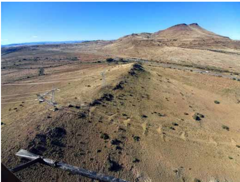
Plate 11: Berms along an access track up a slope to slow runoff and prevent erosion.
