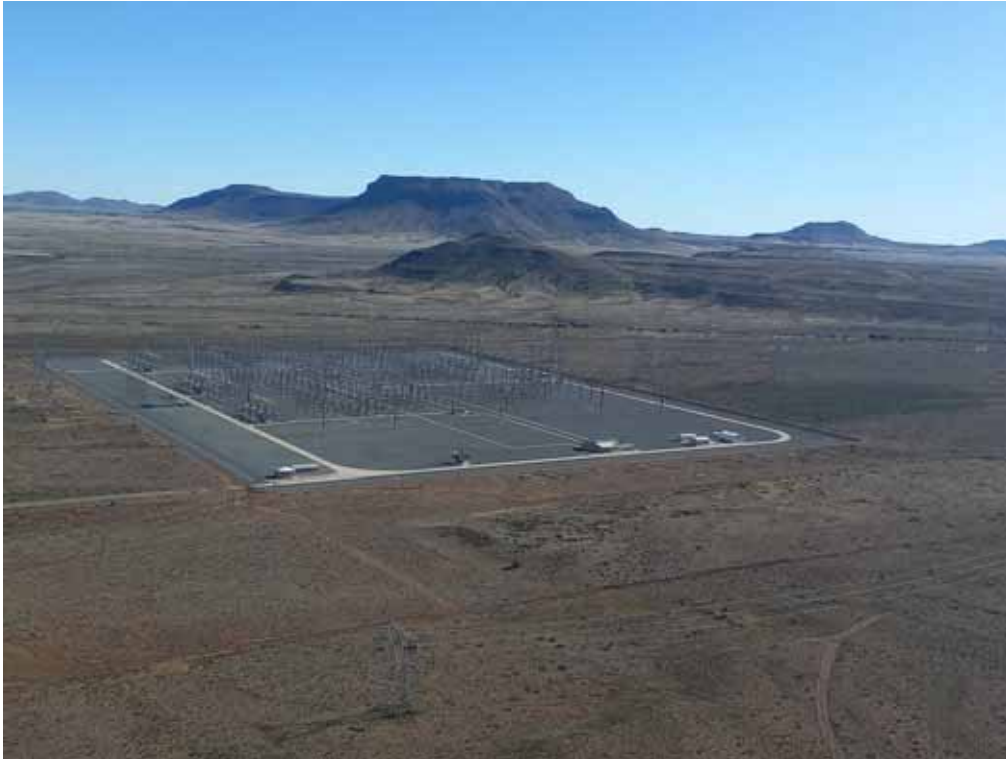
Plate 5: The Gamma Substation and a powerline in the foreground in a flat open plan, with koppies and mesas in the background.
