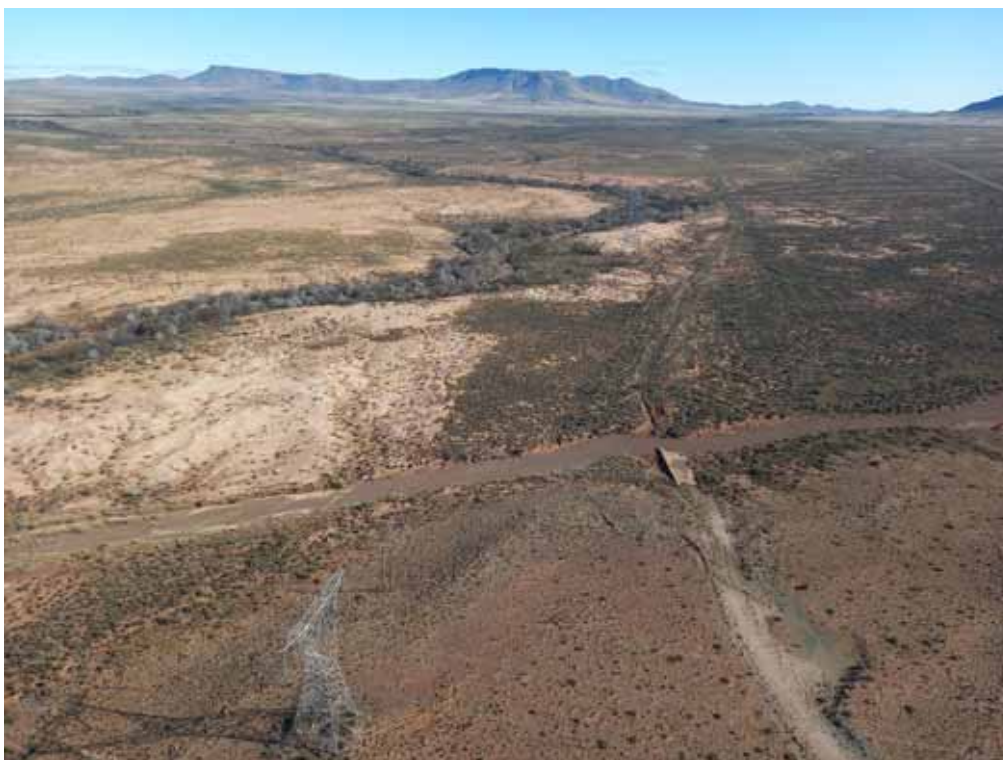
Plate 8: An existing track over a drainage line that has been washed away. High rainfall occurred just prior to the photograph being taken (i.e. July 2022). Access roads over drainage lines need careful placement and design.
