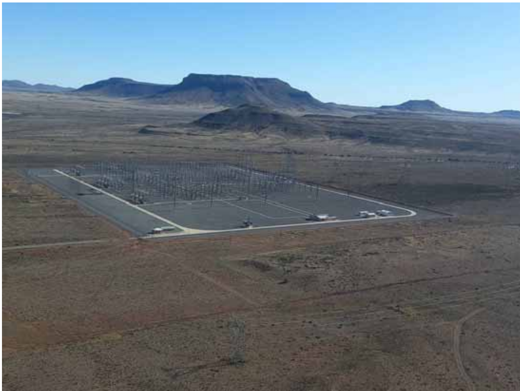
A view of the existing Gamma Substation.
