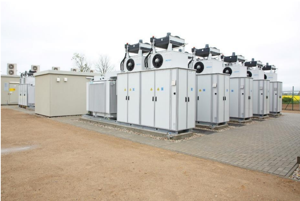
Figure 4.8: Li-Ion BESS containerised modules located within the BESS enclosure footprint (Source: Enel Green Power).
