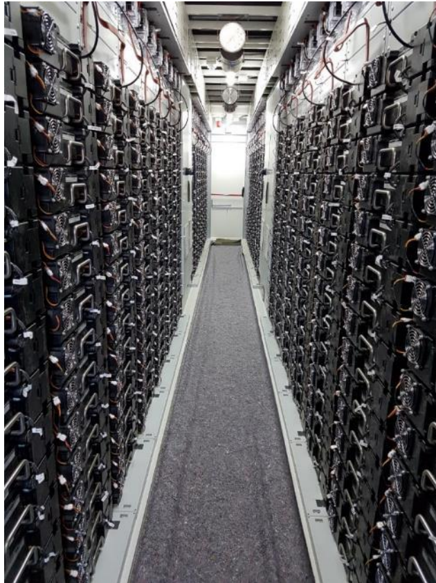
Figure 4.9: Li-Ion BESS internal design and implementation of a container used within a BESS. The image shows a series of sealed battery cell packs within a containerised module (Source: Enel Green Power).
