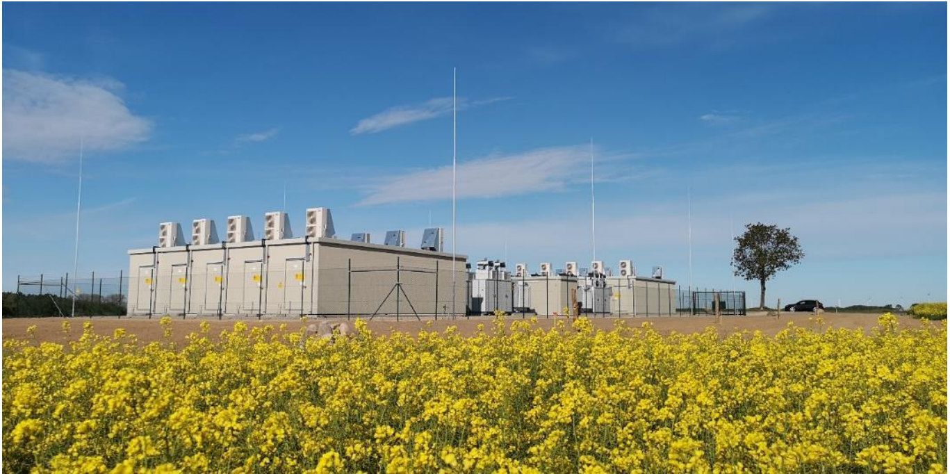
Figure 4.7: Li-Ion BESS implementation for a Renewable Energy facility (Source: Enel Green Power).
