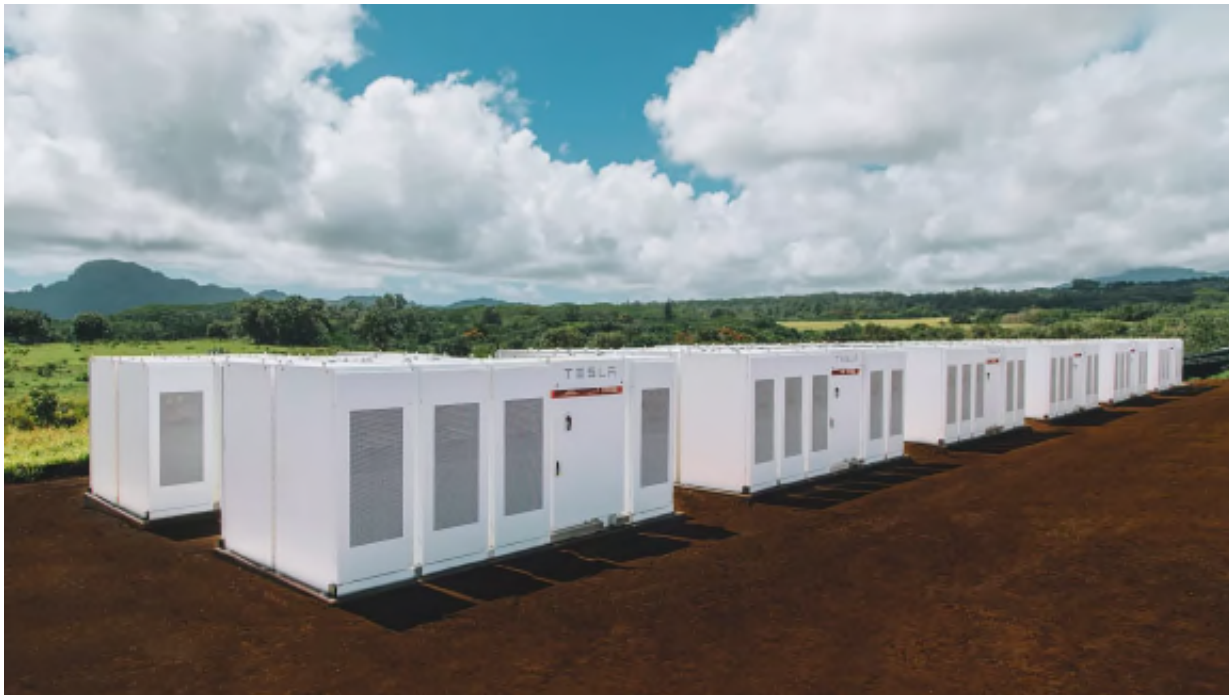
Figure 2.9: Example of battery storage units installed by Tesla (Source: fastcompany.com).
