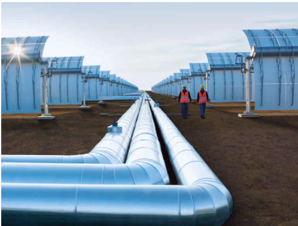
Figure 2.2: The pipes lain between the troughs convey the heat transfer fluid (Source: Siemens AG).
