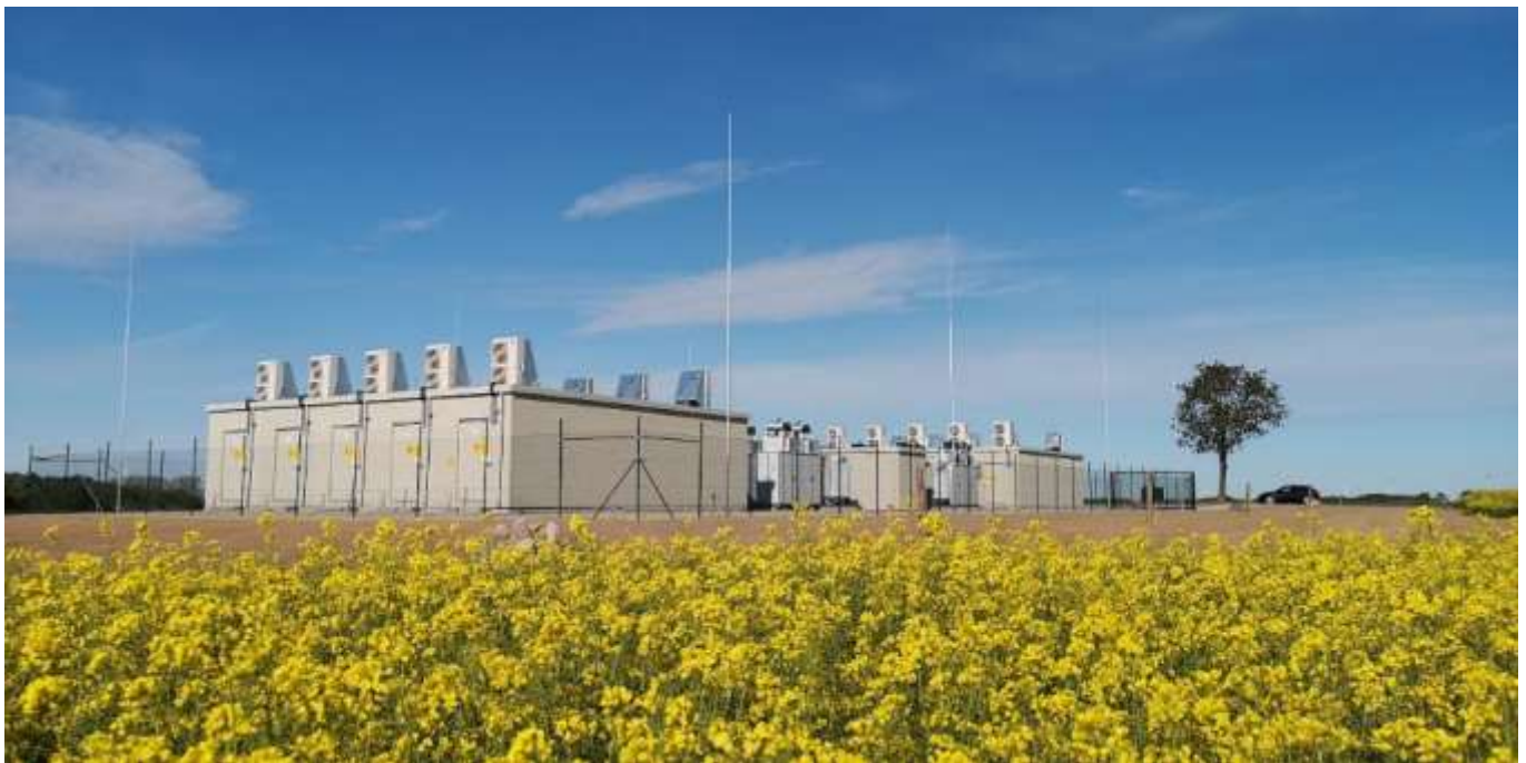
Figure 4.4: Li-Ion BESS implementation for a Renewable Energy facility (Source: Enel Green Power)
