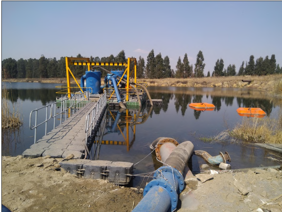
Figure 2.3: Photograph showing the floating jetty/pump used at present to pump water from the Final Cut-off Dam to the Cooling Towers of the power station. The project site identified for the installation of the RO Plant is located to the west of this location.
