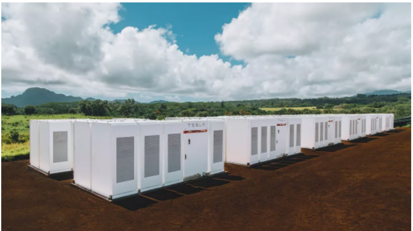
Figure 2.4: Illustration of battery storage units installed by Tesla (Source: fastcompany.com)).
