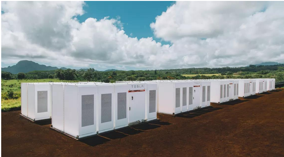
Figure 2.5: Example of battery storage units installed by Tesla (Source: fastcompany.com)
