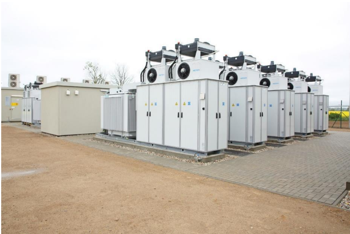
Figure 4.5: Li-Ion BESS containerised modules located within the BESS enclosure footprint (Source: Enel Green Power)
