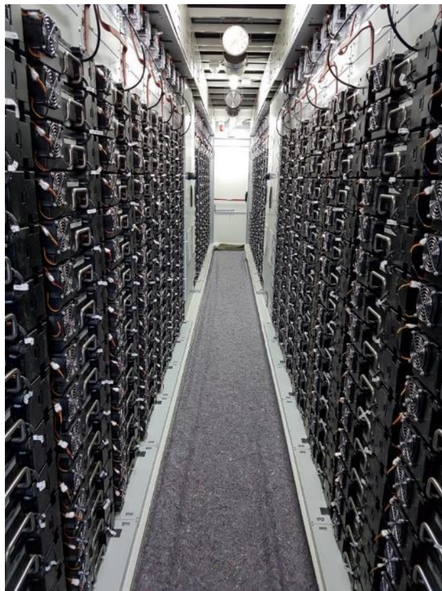
Figure 4.6: Li-Ion BESS internal design and implementation of a container used within a BESS. The image shows a series of sealed battery cell packs within a containerised module (Source: Enel Green Power)
