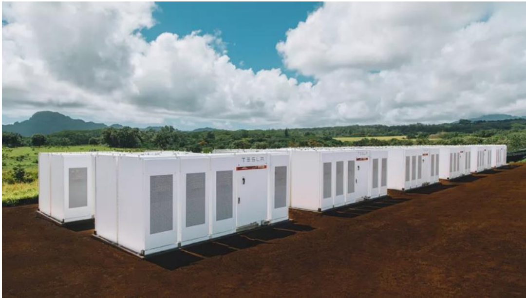
Figure 4.7: Illustration of battery storage units installed by Tesla (Source: fastcompany.com)
