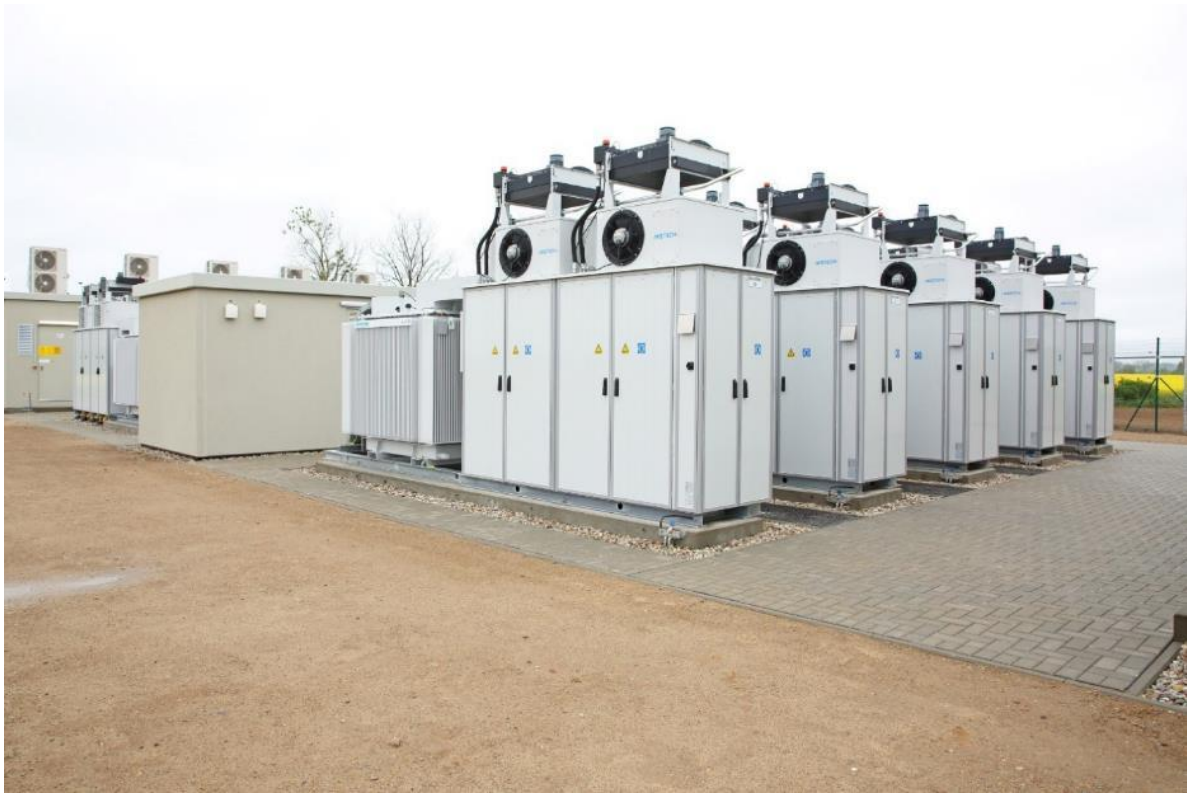
Figure 4.5: Li-Ion BESS containerised modules located within the BESS enclosure footprint (Source: Enel Green Power)
