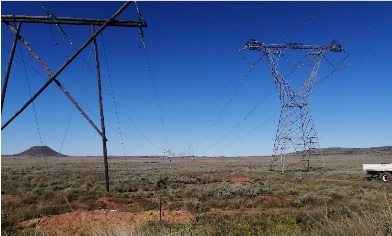
Figure 5.21: Electrical infrastructure that traverses the study area
