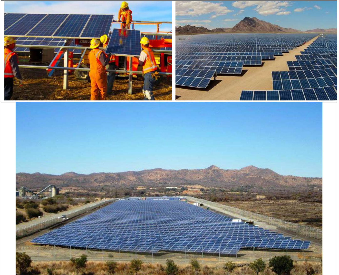
Figure 2.7: Photographs of the construction phase of a solar facility similar to the Harmony One Plant Solar PV Facility
