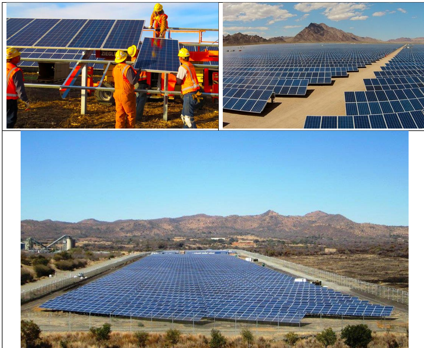
Figure 2.7: Photographs of the construction phase of a solar facility similar to the Harmony Target Solar PV Facility
