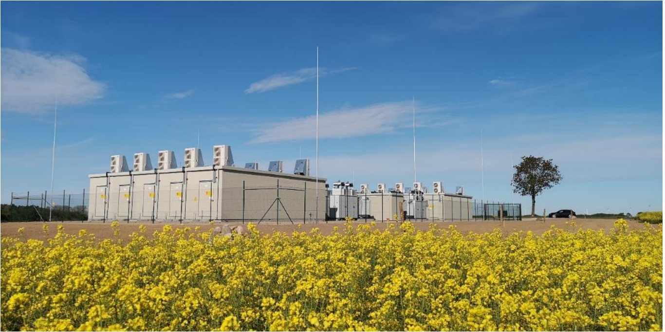
Figure 4.7: Li-Ion BESS implementation for a Renewable Energy facility (Source: Enel Green Power).
