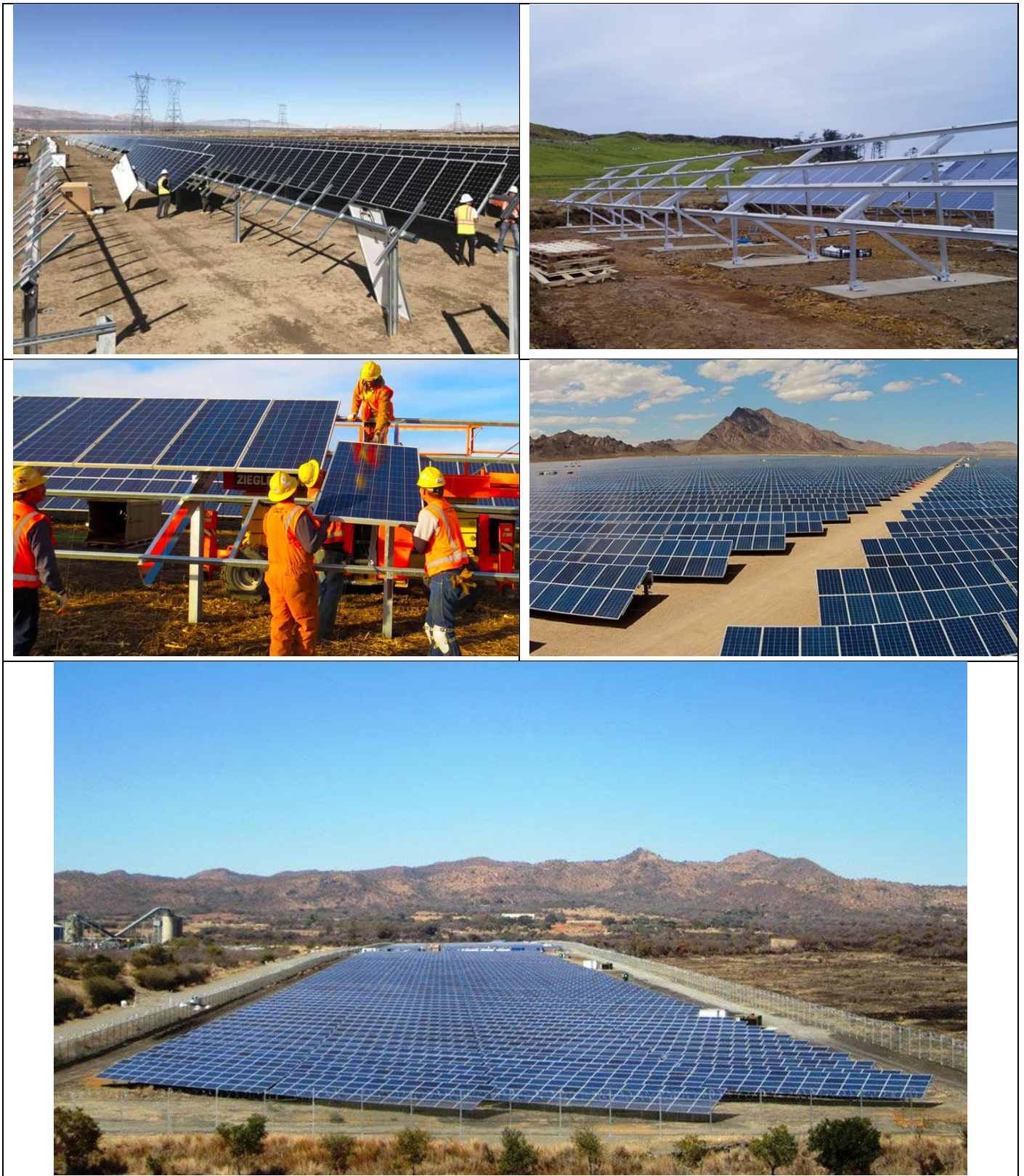
Figure 2.7: Photographs of the construction phase of a solar facility similar to the Highveld Solar PV Facility (Source: https://medium.com/@solar.dao/how-to-build-pv-solar-plant-6c9f6a01020f ; https://www.shutterstock.com/video/clip-1028794-workers-mounting-panels-on-solar-power-plant-construction ; https://www.esi-africa.com/renewable-energy/kenya-construction-solar-farm-gets-green-light/ )
