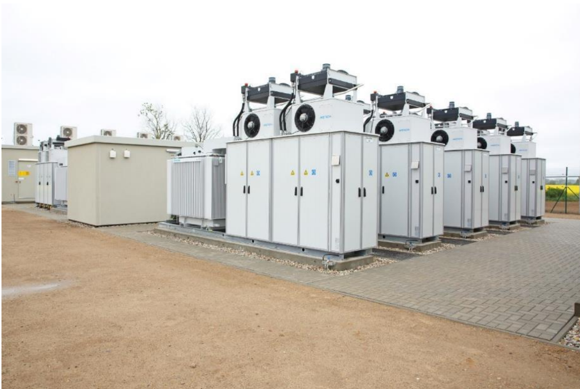
Figure 4.8: Li-Ion BESS containerised modules located within the BESS enclosure footprint (Source: Enel Green Power).
