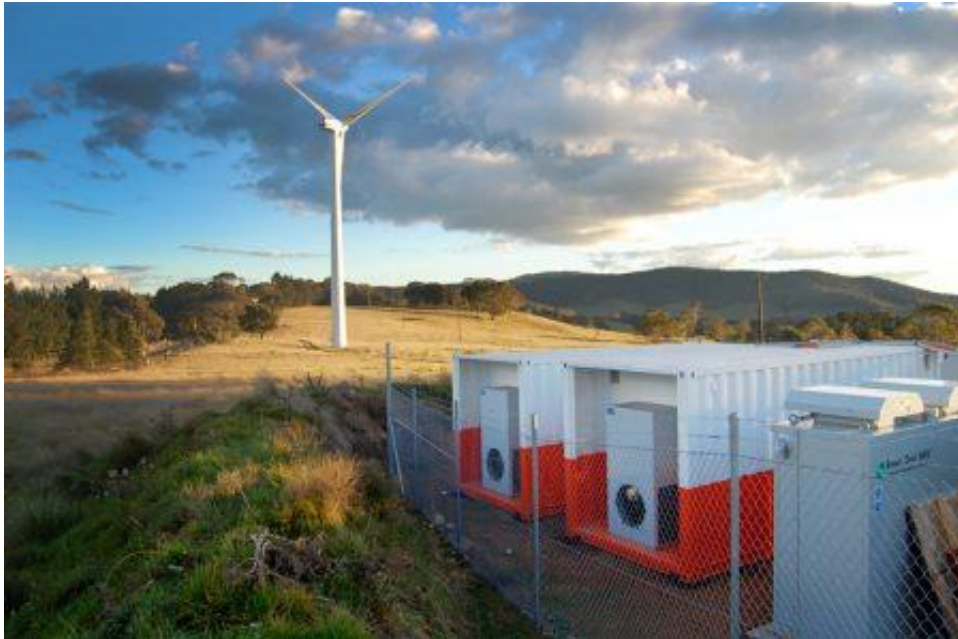
Figure 7.9: Example of battery storage units integrated as part of wind farm (Source: http://ultrabattery.com/applications/stationary-energy-storage/ )
