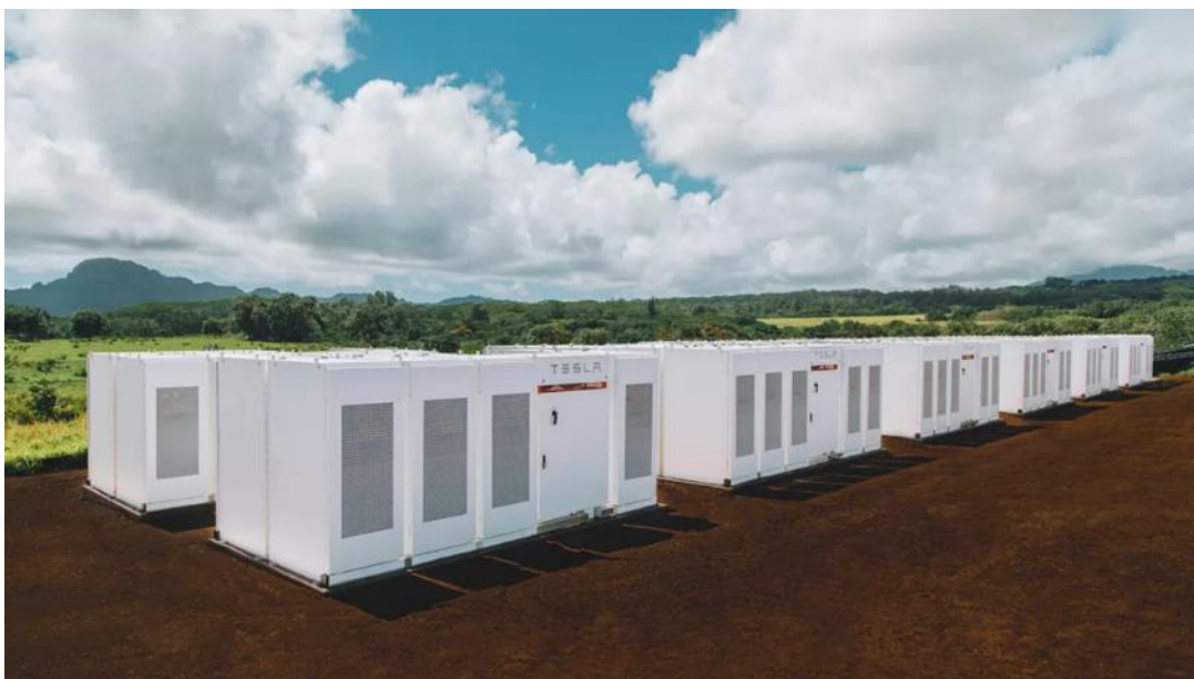
Figure 4.10: Illustration of battery storage units installed by Tesla (Source: fastcompany.com).
