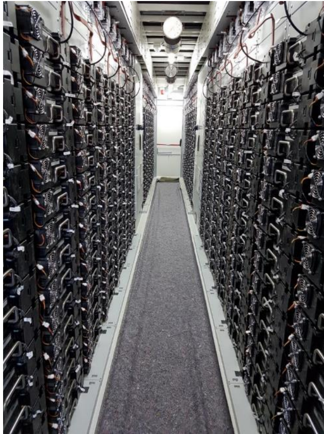
Figure 4.9: Li-Ion BESS internal design and implementation of a container used within a BESS. The image shows a series of sealed battery cell packs within a containerised module (Source: Enel Green Power).
