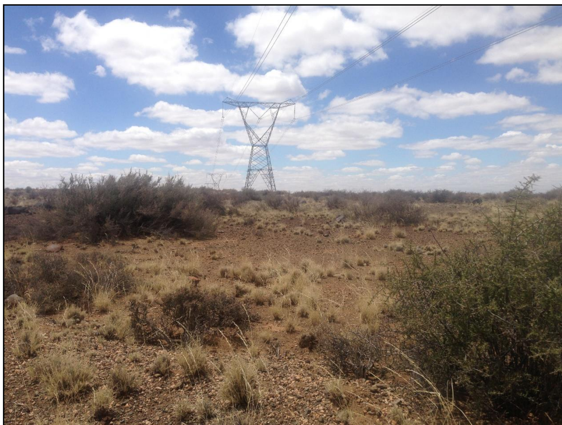
Figure 7.8: Existing Aries/Helios 1 400kV overhead power line.
