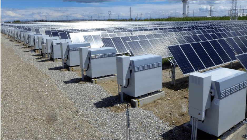
Figure 2.6: Example of battery storage units integrated as part of PV array (Source: nexttracker.com)
