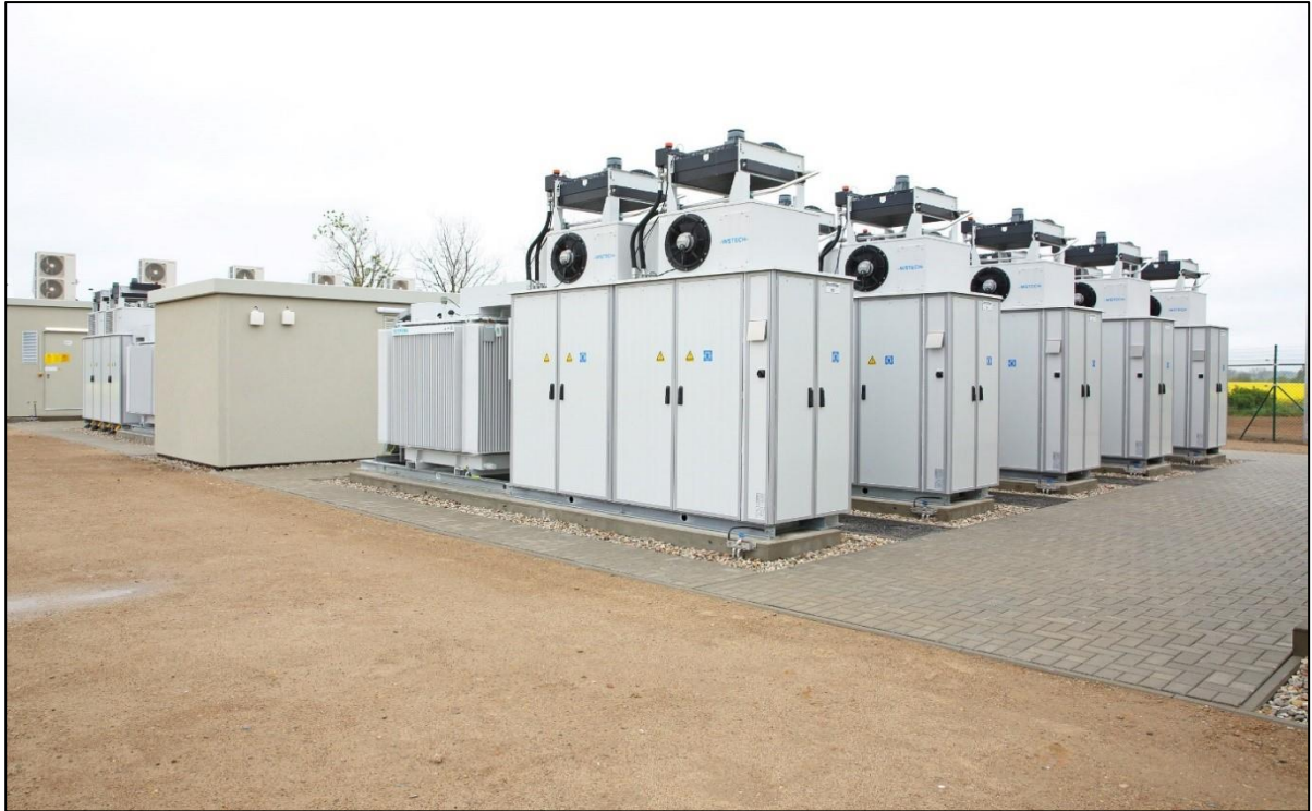
Figure 2.3: Li-Ion BESS containerised modules located within the BESS enclosure footprint (Source: Enel Green Power).
