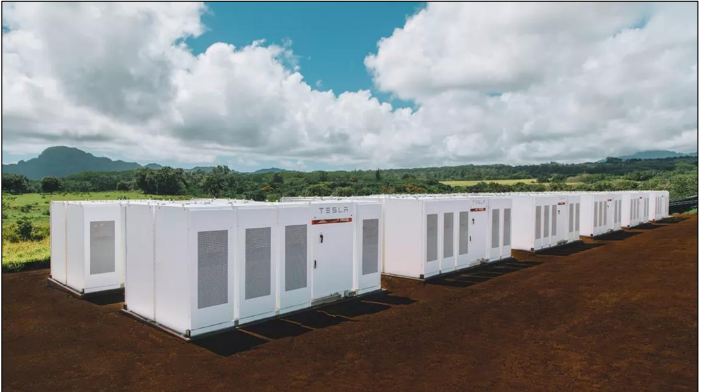
Figure 2.5: Illustration of battery storage units installed by Tesla (Source: fastcompany.com).
