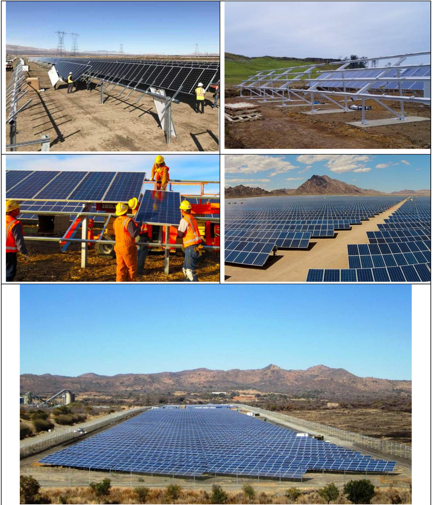
Figure 2.6: Photographs of the construction phase of a solar facility similar to those proposed (Source: https://medium.com/@solar.dao/how-to-build-pv-solar-plant-6c9f6a01020f ; https://www.shutterstock.com/video/clip-1028794-workers-mounting-panels-on-solar-power-plant-construction ; https://www.esi-africa.com/renewable-energy/kenya-construction-solar-farm-gets-green-light/ ).
