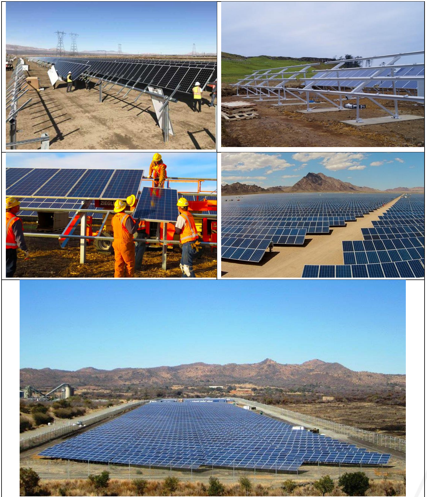
Figure 4.4: Photographs of the construction phase of a solar facility similar to those proposed
