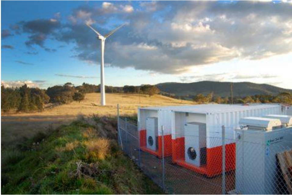
Figure 8.7 Example of battery storage units integrated as part of wind farm (Source: http://ultrabattery.com/applications/stationary-energy-storage/ )
