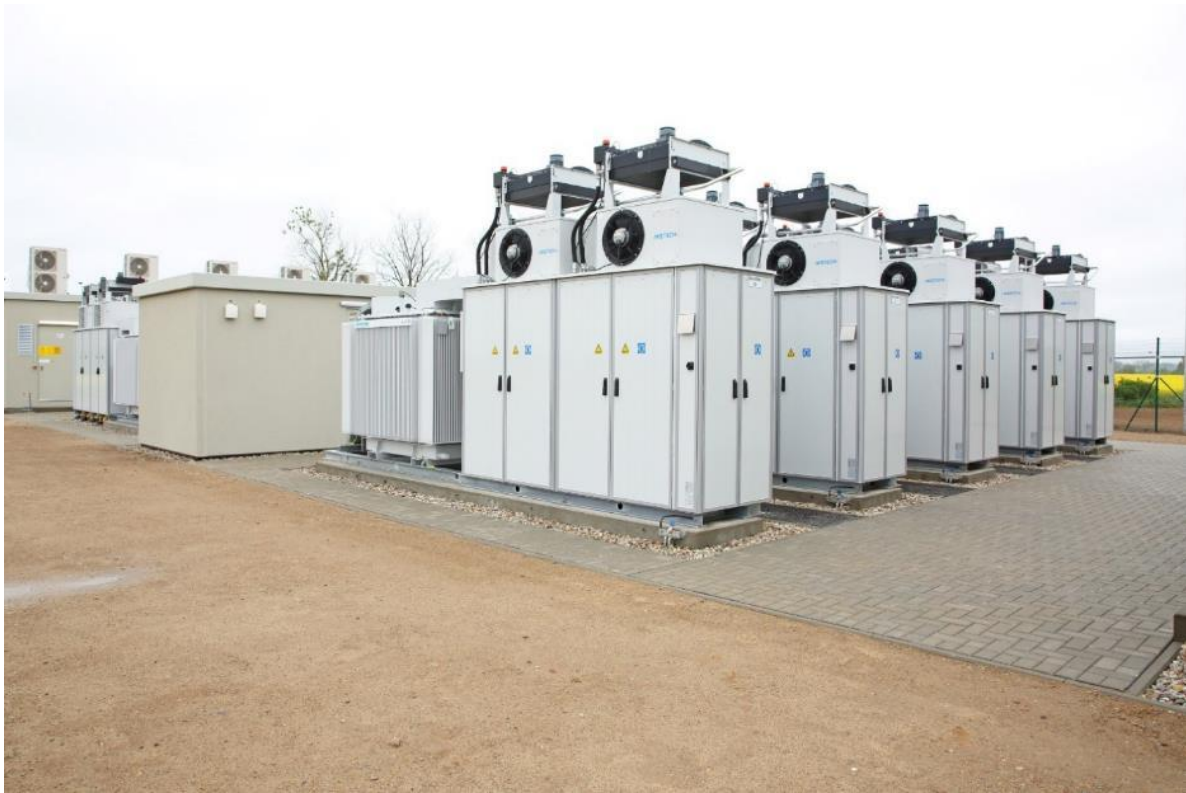
Figure 4.10: Li-Ion BESS containerised modules located within the BESS enclosure footprint (Source: Enel Green Power)
