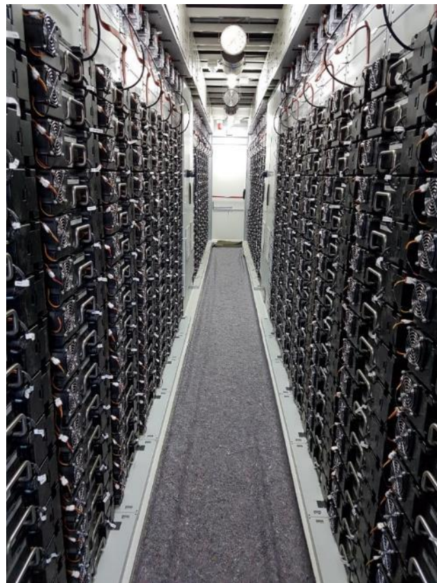
Figure 4.11: Li-Ion BESS internal design and implementation of a container used within a BESS. The image shows a series of sealed battery cell packs within a containerised module (Source: Enel Green Power)
