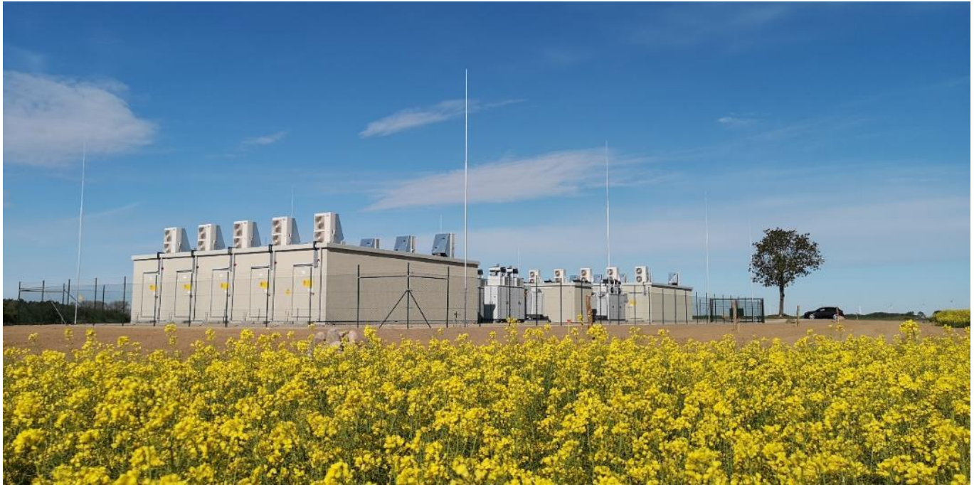
Figure 2.6: Li-Ion BESS implementation for a Renewable Energy facility (Source: Enel Green Power)
