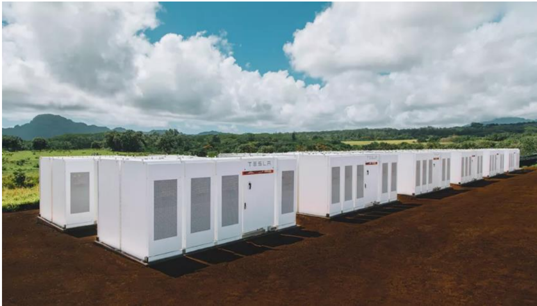
Figure 4.12: Illustration of battery storage units installed by Tesla (Source: fastcompany.com)
