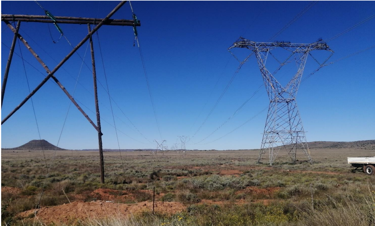
Figure 5.21: Electrical infrastructure that traverses the study area
