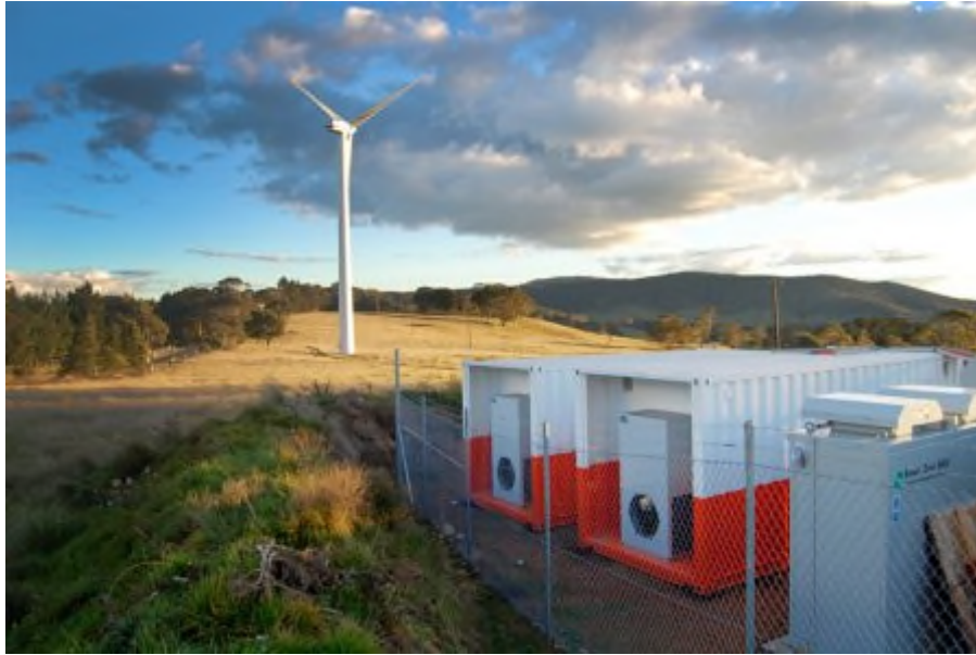
Figure 9.12: Example of battery storage units integrated as part of a wind farm (Source: http://ultrabattery.com/applications/stationary-energy-storage/ )
