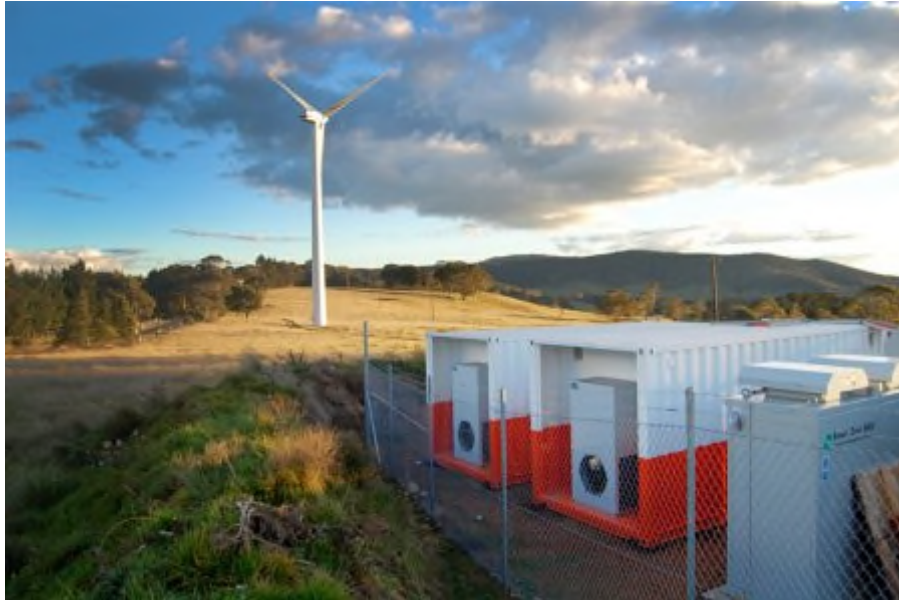
Figure 9.12: Example of battery storage units integrated as part of a wind farm (Source: http://ultrabattery.com/applications/stationary-energy-storage/ )
