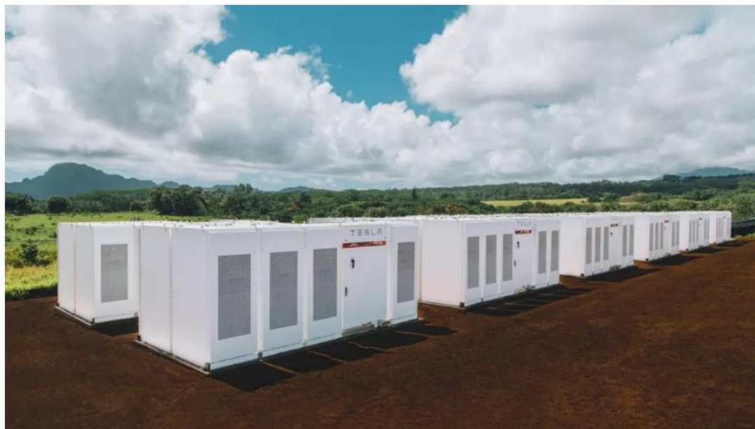
Figure 2.12: Illustration of battery storage units installed by Tesla (Source: fastcompany.com).
