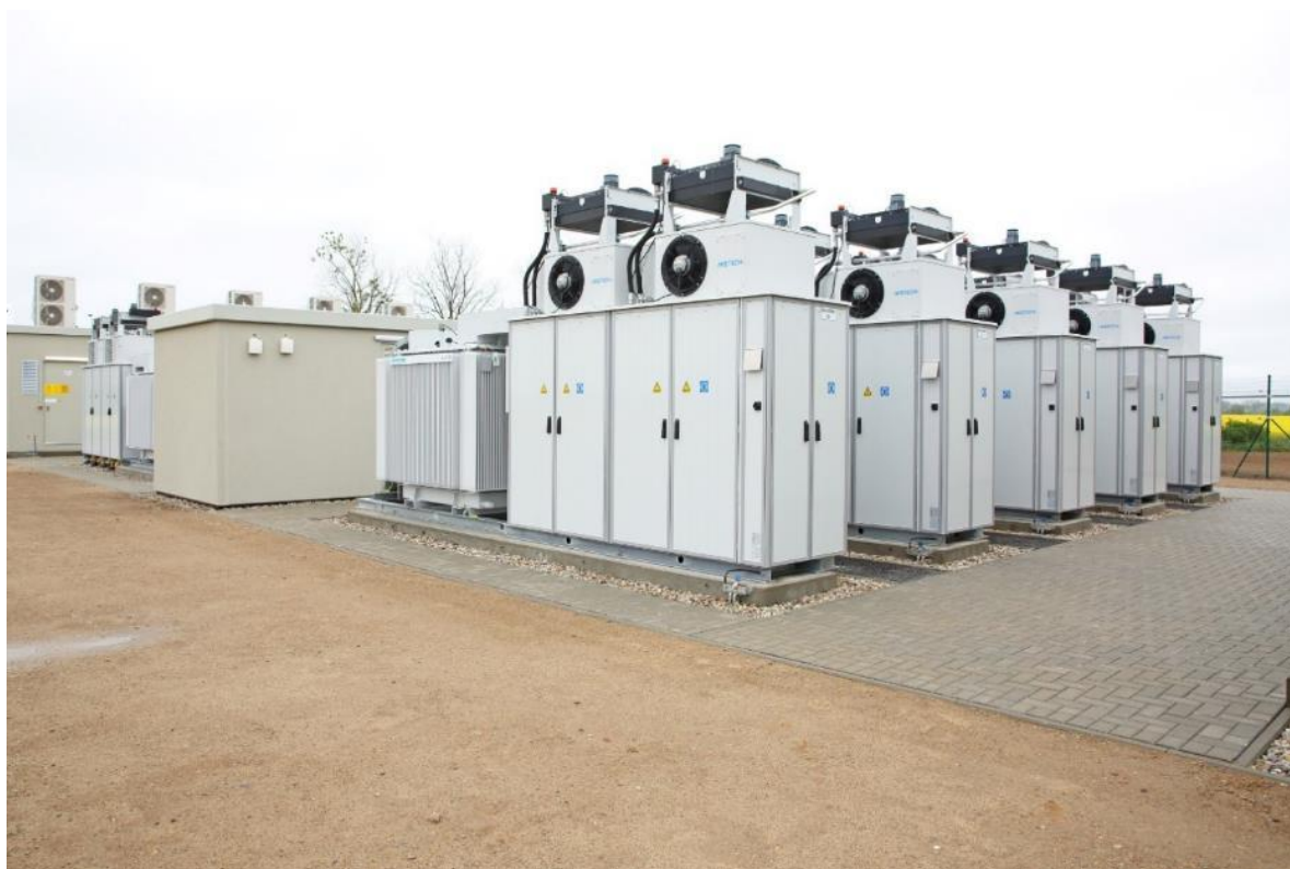
Figure 2.10: Li-Ion BESS containerised modules located within the BESS enclosure footprint (Source: Enel Green Power).
