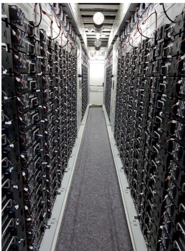
Figure 2.11: Li-Ion BESS internal design and implementation of a container used within a BESS. The image shows a series of sealed battery cell packs within a containerised module (Source: Enel Green Power).
