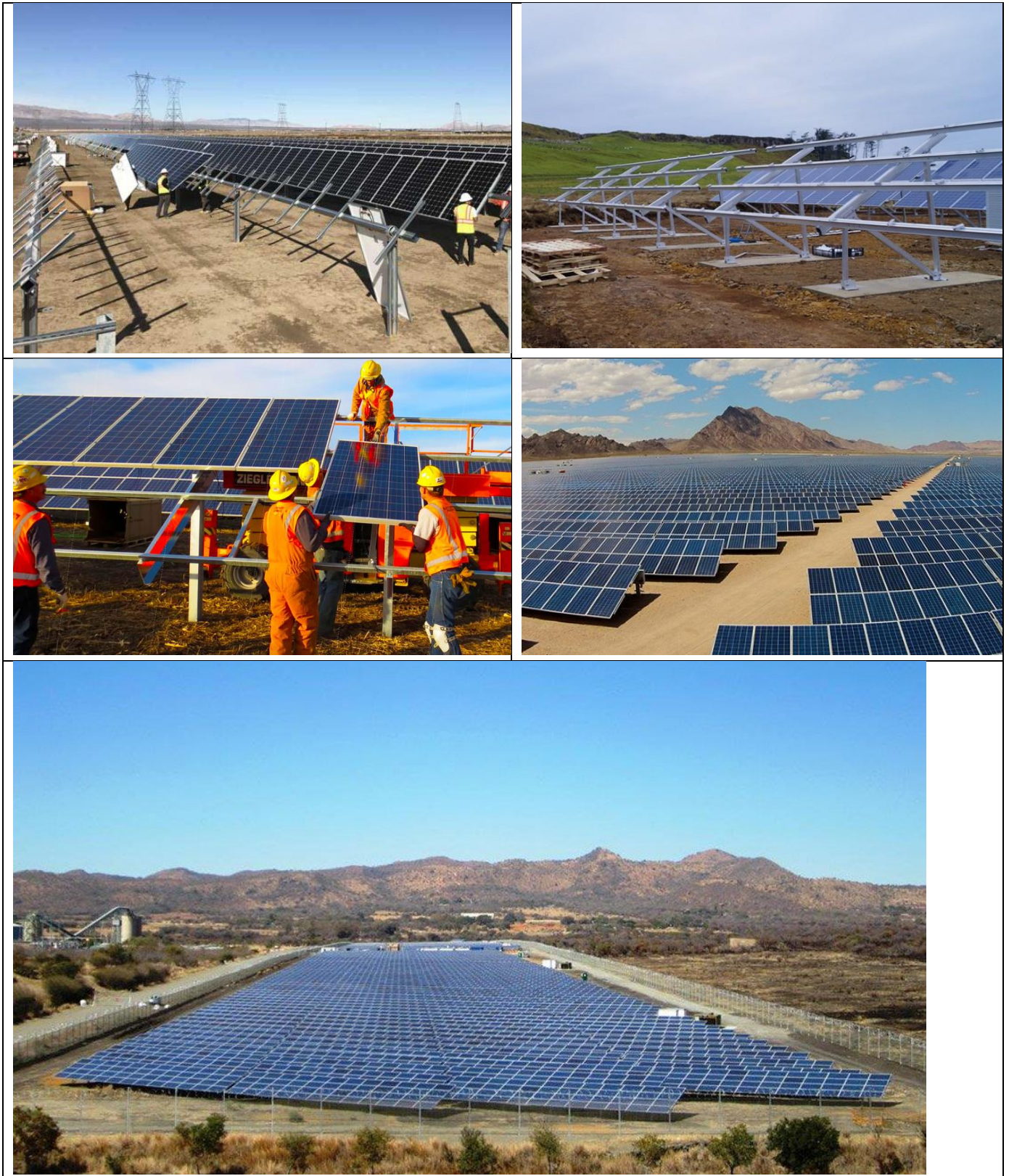
Figure 4.1: Photographs of the construction phase of a solar facility similar to those proposed
