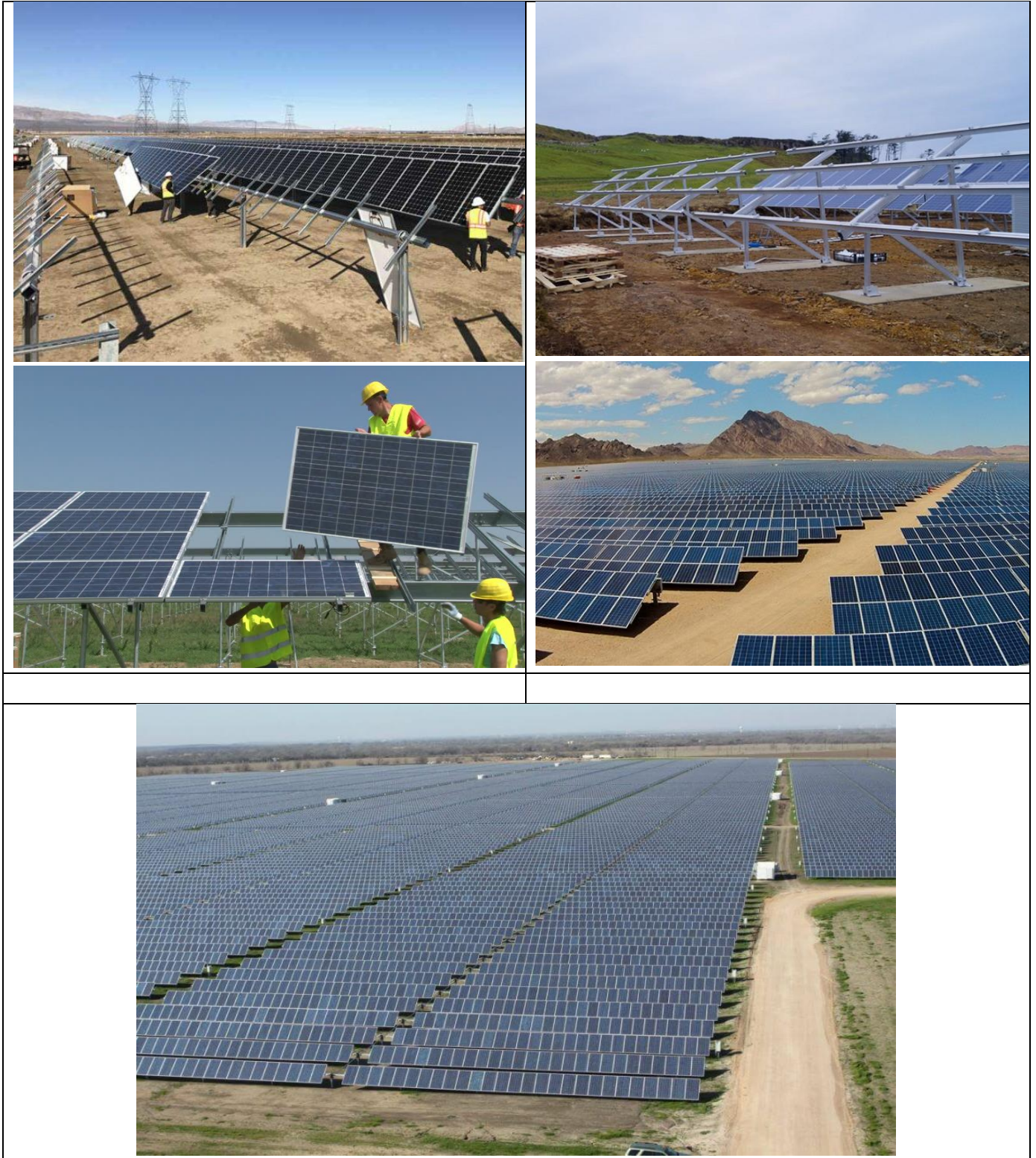
Figure 2.11: Photographs of the construction phase of a Solar Energy Facility similar to the Project (Source: https://medium.com/@solar.dao/how-to-build-pv-solar-plant-6c9f6a01020f ; https://www.shutterstock.com/video/clip-1028794-workers-mounting-panels-on-solar-power-plant-construction ; https://www.esi-africa.com/renewable-energy/kenya-construction-solar-farm-gets-green-light/ )
