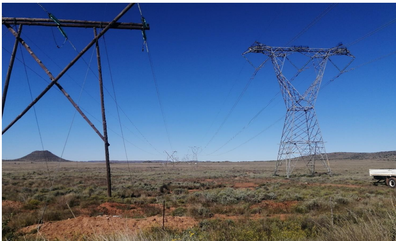
Figure 5.21: Electrical infrastructure that traverses the study area
