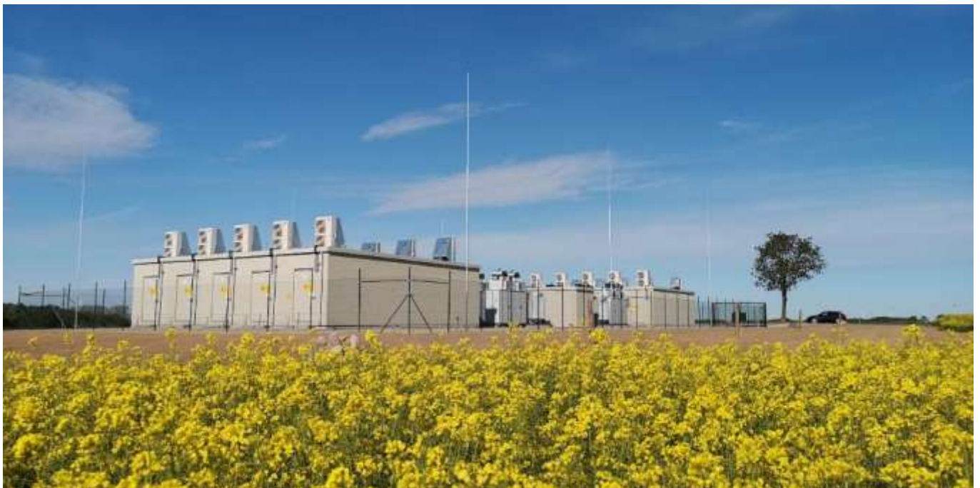
Figure 4.4: Li-Ion BESS implementation for a Renewable Energy facility (Source: Enel Green Power)
