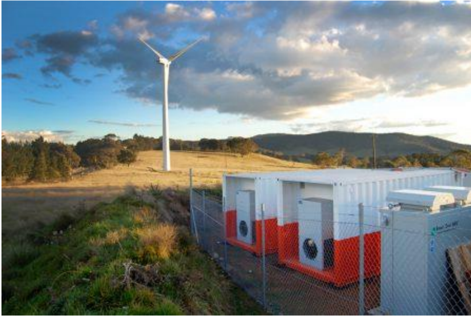
Figure 9.11: Example of battery storage units integrated as part of solar facility (Source: http://ultrabattery.com/applications/stationary-energy-storage/ )
