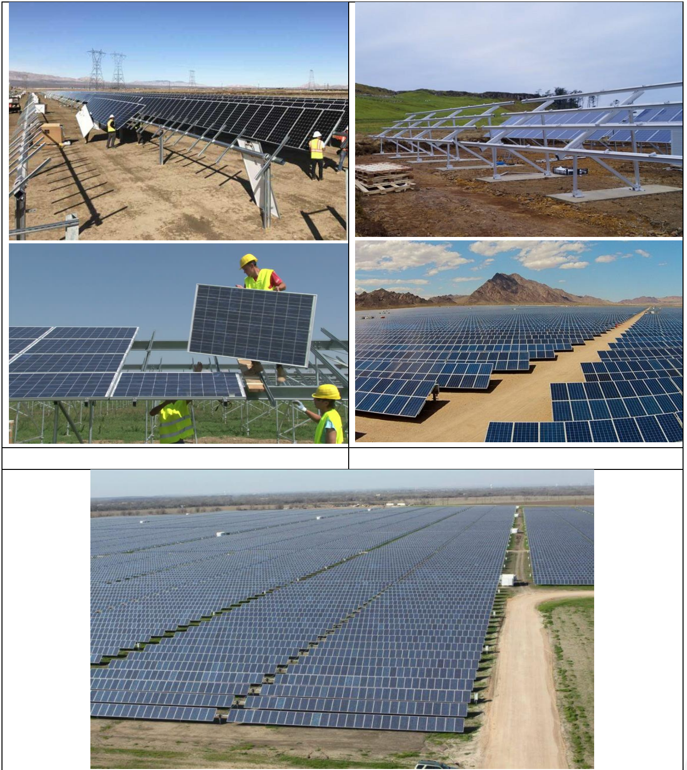
Figure 2.8: Photographs of the construction phase of a Solar Energy Facility similar to the Project (Source: https://medium.com/@solar.dao/how-to-build-pv-solar-plant-6c9f6a01020f ; https://www.shutterstock.com/video/clip-1028794-workers-mounting-panels-on-solar-power-plant-construction ; https://www.esi-africa.com/renewable-energy/kenya-construction-solar-farm-gets-green-light/ )
