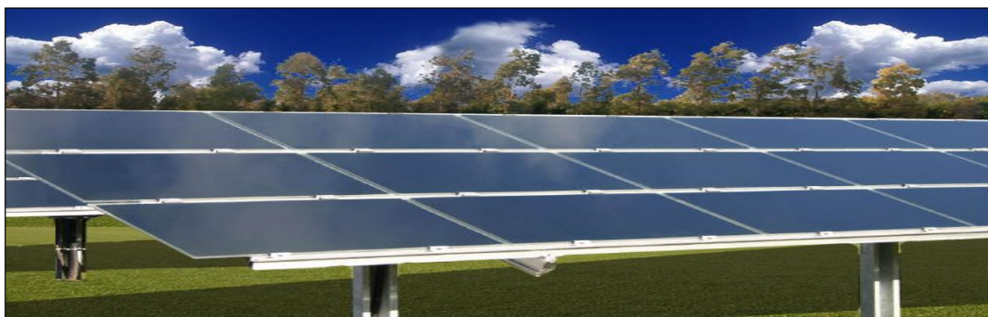
Figure 5-3. Frontal views of PV arrays mounted on fixed mounting systems.
