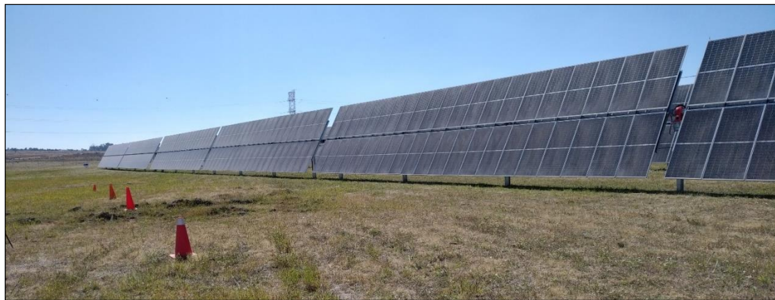
Figure 5-5. Frontal views of PV arrays mounted on fixed mounting systems.
