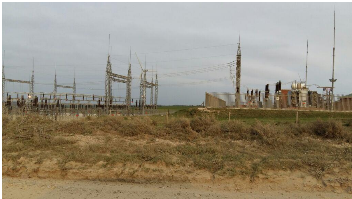
Figure 5.8: Substation / switching station
