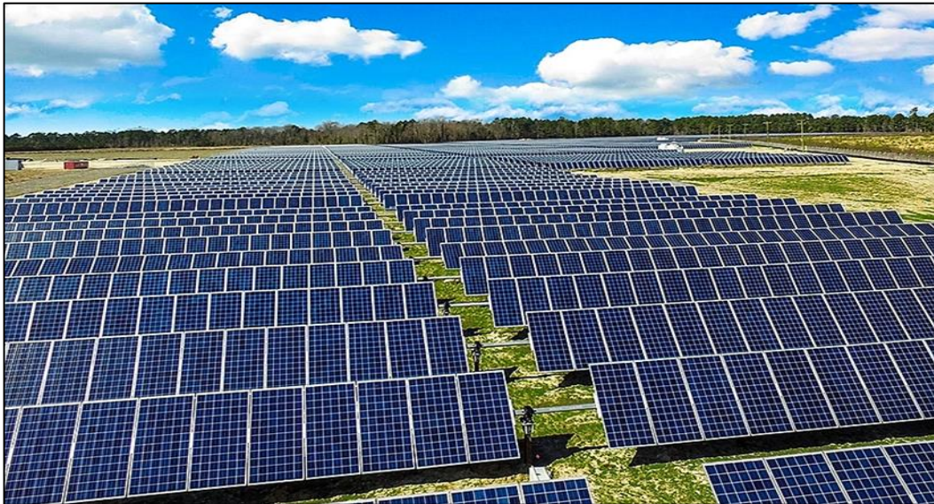
Figure 2-1: Typical example of solar PV array
