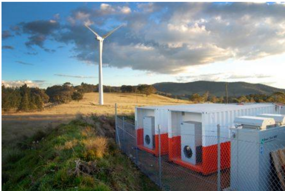
Figure 9.10: Example of battery storage units integrated as part of wind farm (Source: http://ultrabattery.com/applications/stationary-energy-storage/ )
