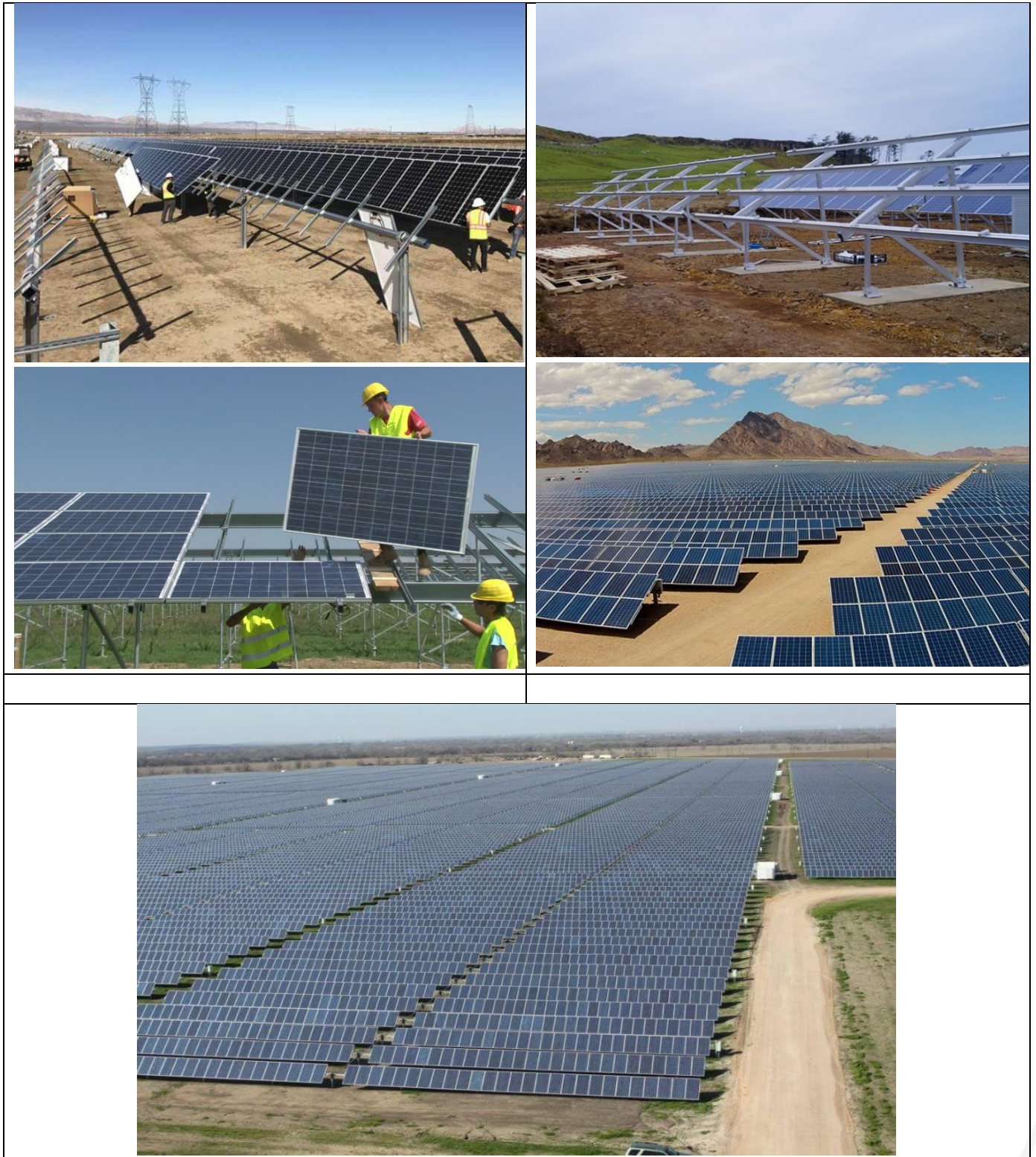
Figure 2.3: Photographs of the construction phase of a Solar Energy Facility similar to Mutsho PV1 (Source: https://medium.com/@solar.dao/how-to-build-pv-solar-plant-6c9f6a01020f ; https://www.shutterstock.com/video/clip-1028794-workers-mounting-panels-on-solar-power-plant-construction ; https://www.esi-africa.com/renewable-energy/kenya-construction-solar-farm-gets-green-light/ )
