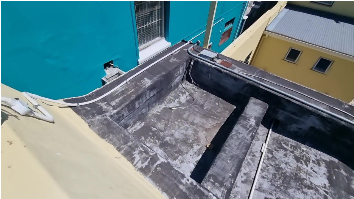
Figure 16: Image shows the parapet waterproofing membrane where the fixing of services seems to penetrate and compromise the waterproofing.
