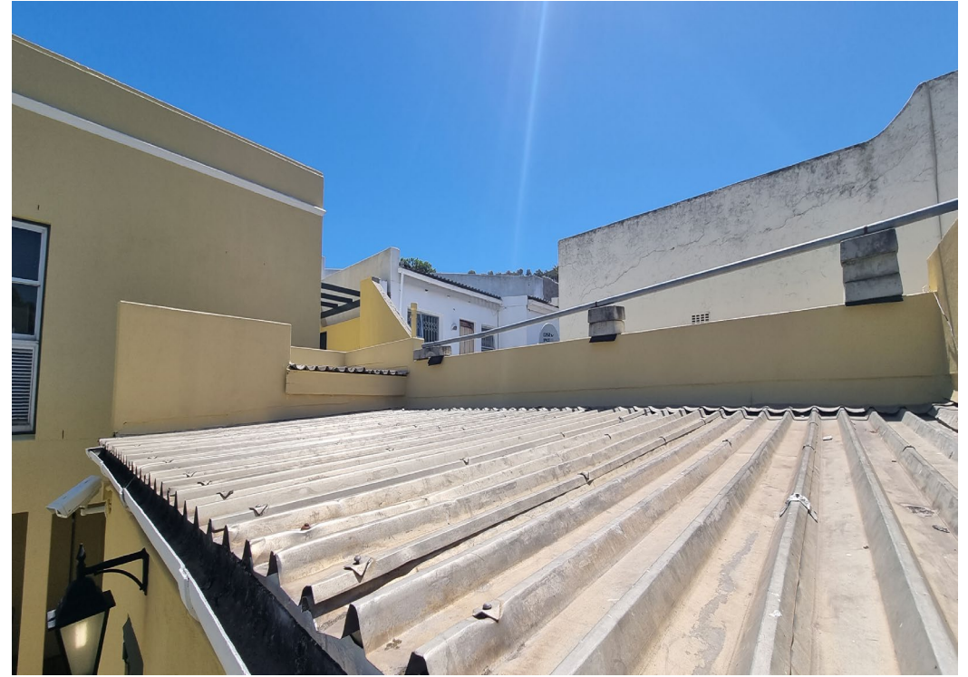
Figure 32: Image shows the roof sheets have a limited lifespan with visible previous repairs and damage to sheets. Replace fixing screws, fit poly closures to end of sheets.
