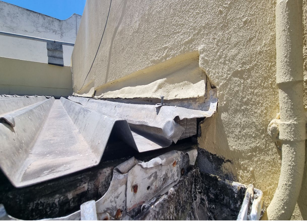
Figure 33: Image shows the roof sheets have a limited lifespan with visible previous repairs and damage to sheets. Replace fixing screws, fit poly closures to end of sheets. Fit new flashings to head and sidewalls.
