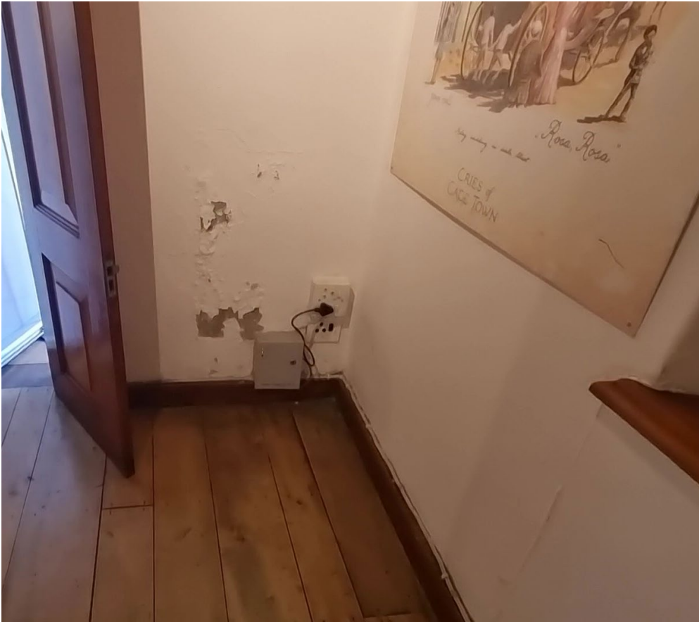
Figure 10: Image shows water damage to a wall in the East-Room (Exhibition room 3).
