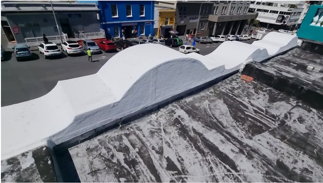
Figure 13: Image shows the gable end parapet waterproofing seem to be in good condition.
