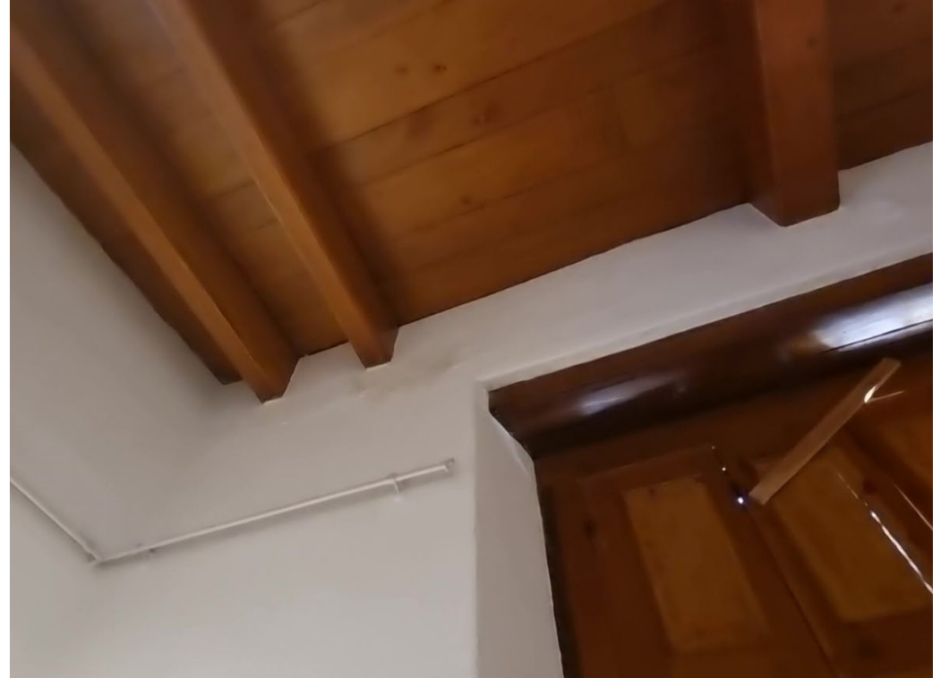
Figure 11: Image shows water damage to the underside of the ceiling.
