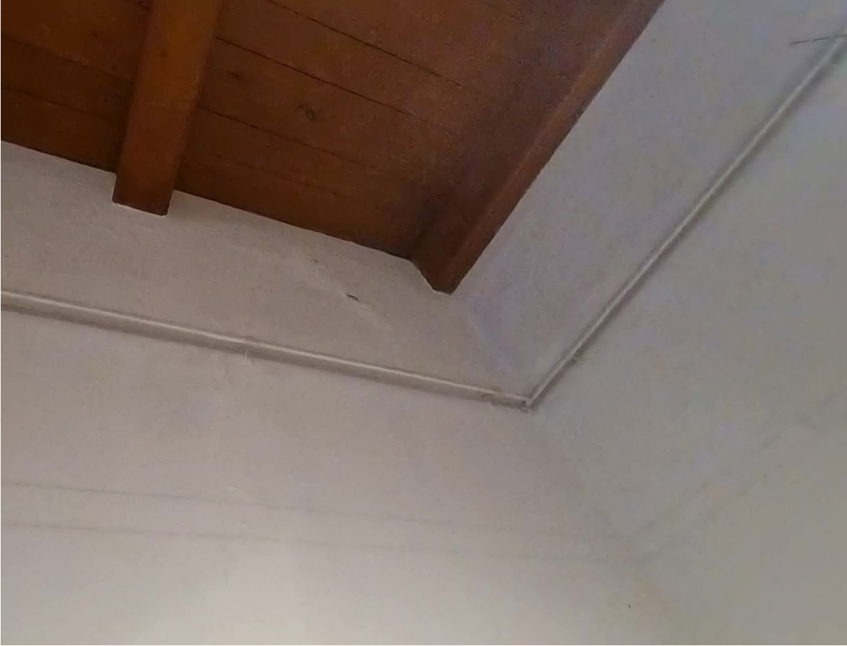
Figure 12: Image shows water damage to the walls and ceiling.
