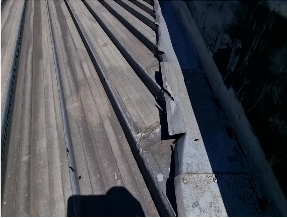
Figure 25: Image shows noticeable damaged flashing and extended sheets with rivets. New Flashing recommended.
