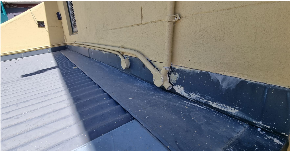
Figure 36: Image shows visible damage to headwall flashing and retrofitted services penetrating plate and compromising water ingress.
