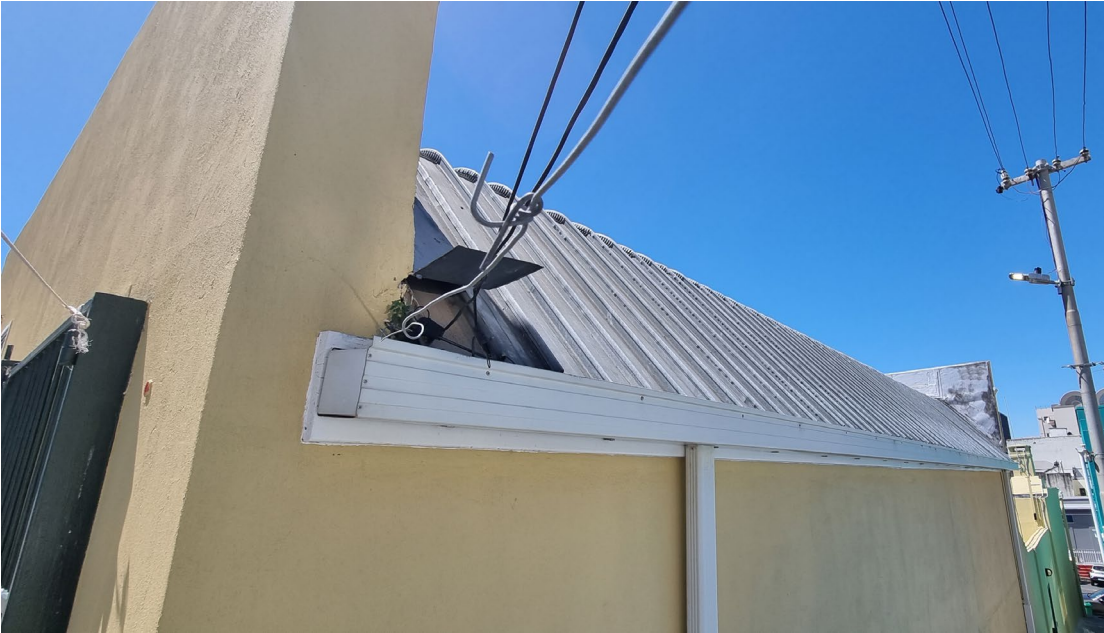
Figure 23: Image shows damaged sidewall flashing on angled return.
