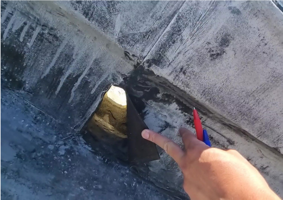
Figure 19: Image shows compromised Torch on waterproofing to emergency outlet. Patch and service this area.
