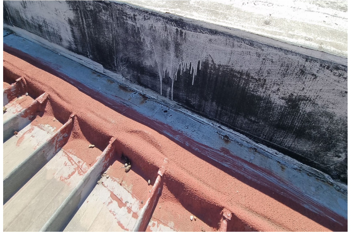
Figure 26: Image shows poor application of incorrect product. New flashing recommended.
