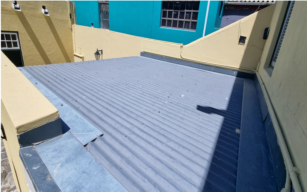
Figure 22: Image shows roof to be in fair condition but visible damage to headwall flashing and retrofitted services penetrating plate and compromising water ingress can be seen.
