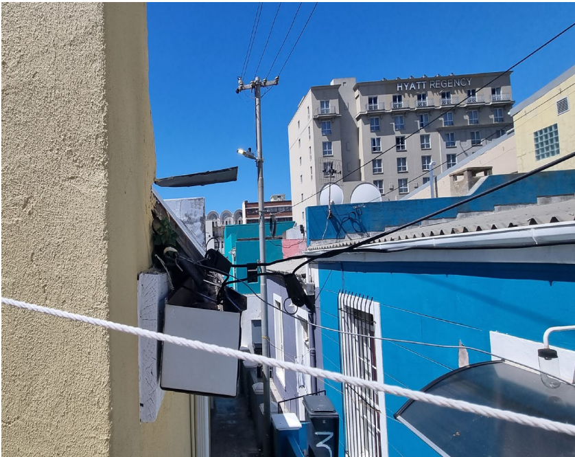
Figure 24: Image shows the exposed roof structure. Custom flashing to close off corner is recommended.
