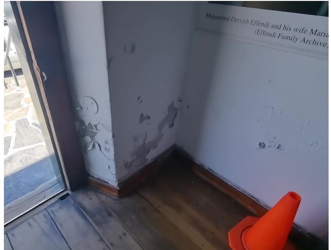
Figure 9: Image shows noticeable damp damage next to front entrance door.
