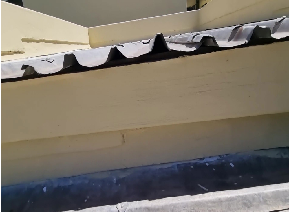
Figure 31: Image shows that the roof sheets has reached the end of lifespan with visible previous repairs and damage to sheets.
