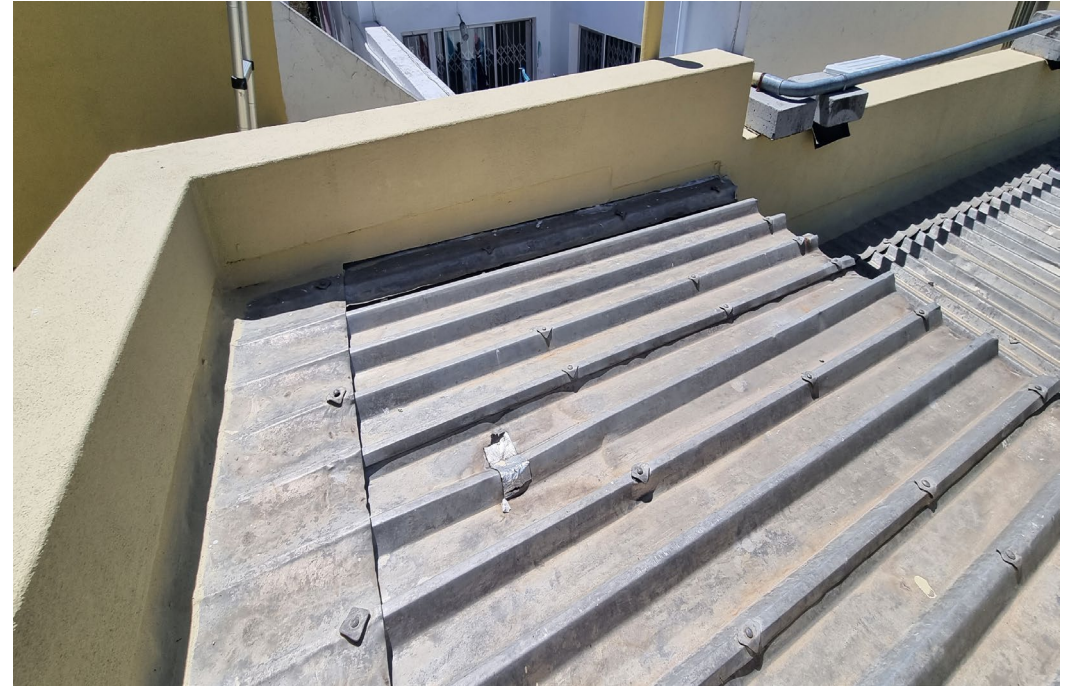
Figure 30: Image shows the roof sheets have reached the end of lifespan with visible previous repairs and damage to sheets.
