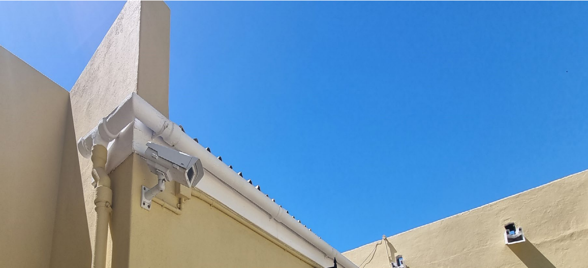
Figure 34: Image shows visible damage to Rainwater goods – replace with fibre cement.
