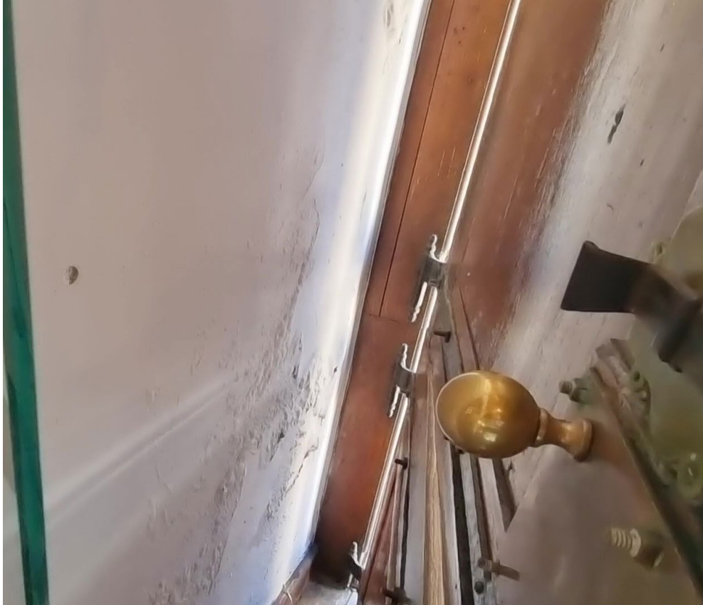
Figure 8: Image shows noticeable damp damage behind front entrance door.
