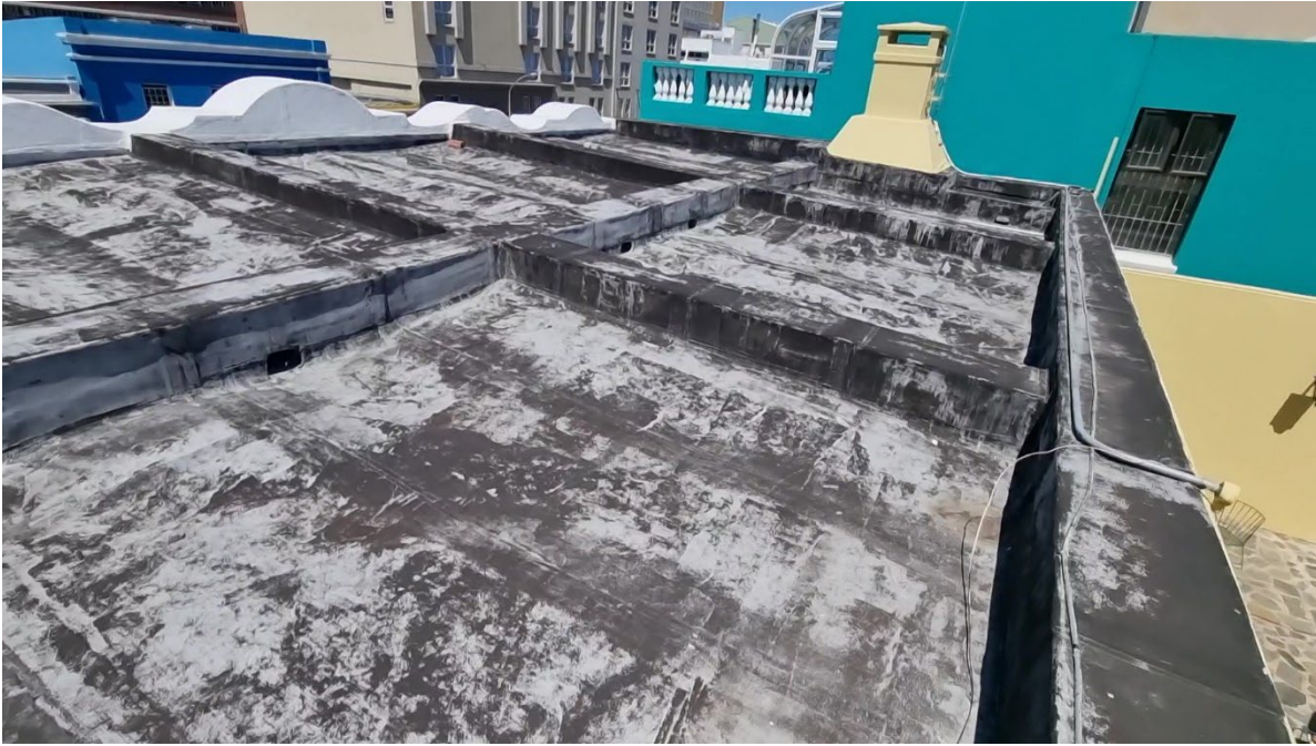
Figure 21: Image shows an overall view of roof indicating wear and exposed torch on membrane.
