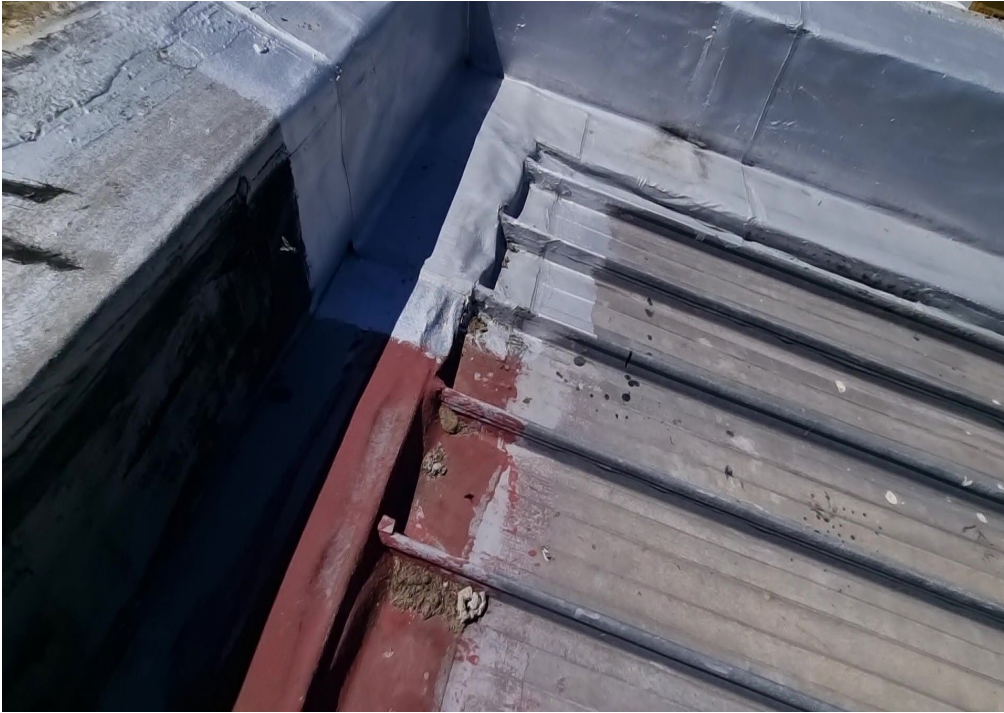
Figure 29: Image shows poor application of incorrect product. New flashing recommended.
