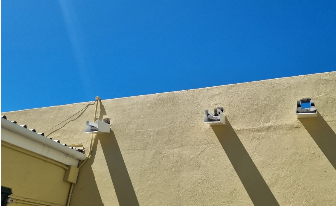
Figure 17: Image shows the water outlets to roof in clean and good condition. Discuss the option of hopper boxes and downpipes.
