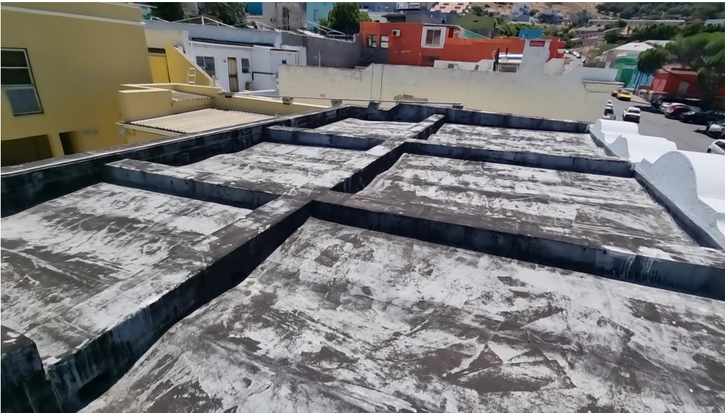
Figure 20: Image shows an overall view of roof indicating wear and exposed torch on membrane.
