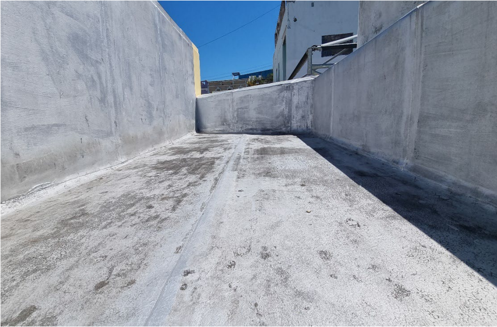
Figure 27: Image shows the flat roof to entrance. Vertical waterproofing in fair condition, but rather replace with new roof.
