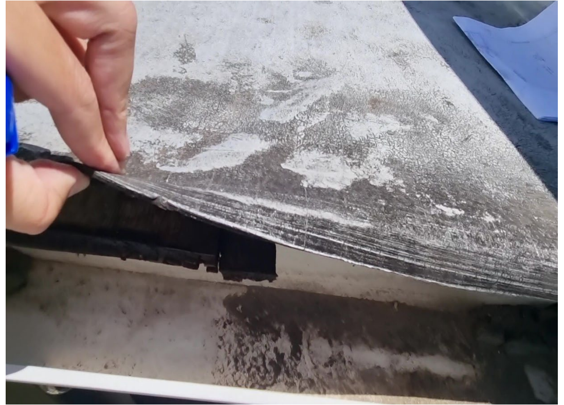
Figure 28: Image shows visible delamination to flat roof with wood rot below. Replace entire roof.
