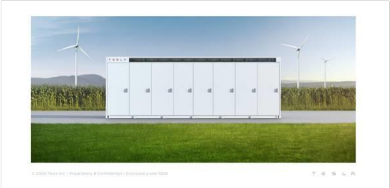
Figure 4.4: Li-Ion BESS containerised modules located within the BESS enclosure footprint (Source: Tesla).
