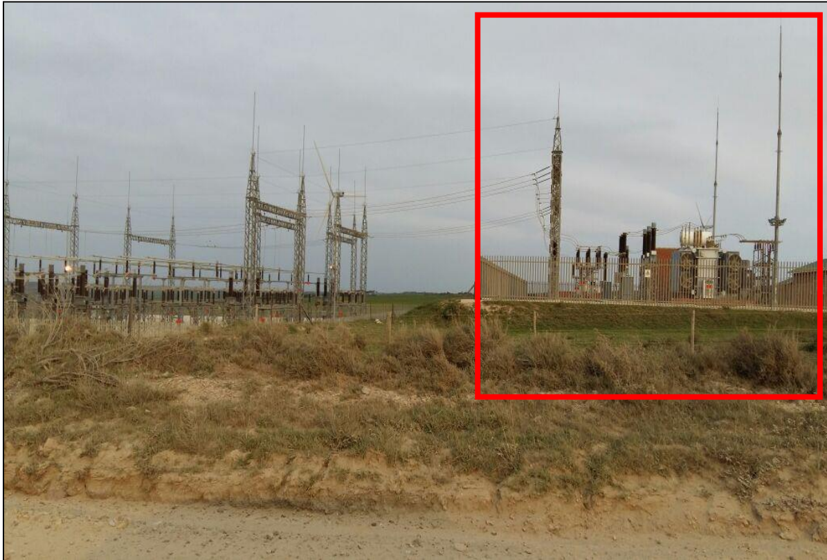
Figure 4: Example of an On-site Substation (Operator portion) (left) and adjoining Wind Facility substation (IPP portion) (right) on the Kouga Wind Facility
