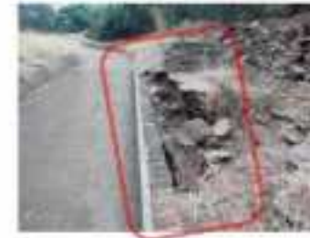
A spill to flow over a spill. This damage was caused by storm-water overflow from the dam. Some more storm-water could destroy the spillway and then the dam.
