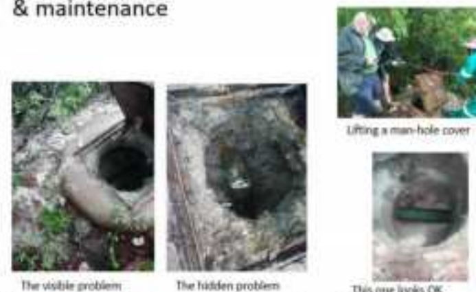
Figure 1: Photographs of the sewage situation at Kloofendal as presented by FroK
