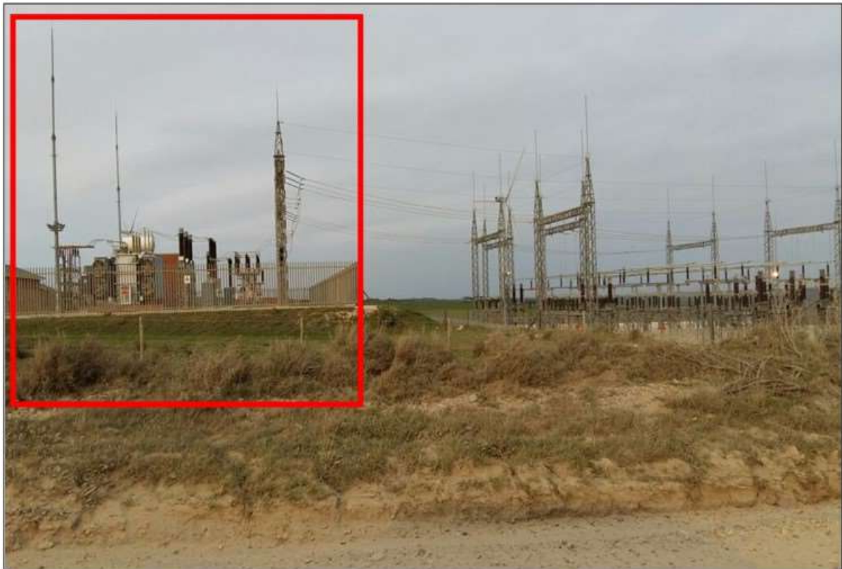
Figure 4: Photograph of the Kouga Wind Energy Facility illustrating the relationship between the on-site substation (IPP Portion) (left) and adjoining grid substation/switching station (Operator Portion)
