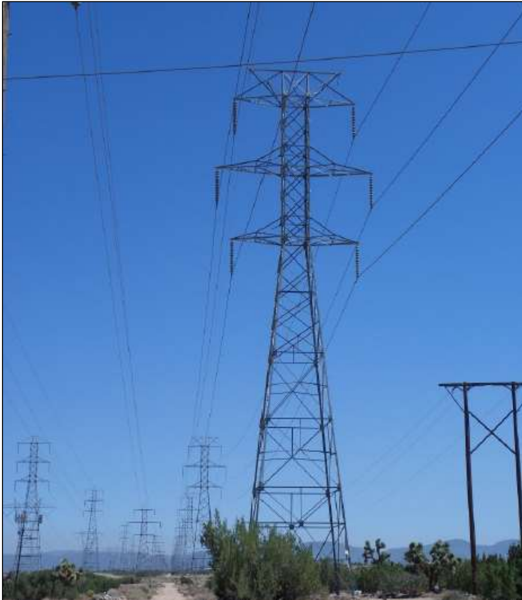
Figure 14: 132kV/275kV Powerline Double Circuit Suspension Towers
