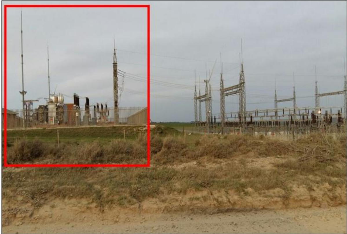
Figure 4: Photograph of the Kouga Wind Energy Facility illustrating the relationship between the on-site substation (IPP Portion) (left) and adjoining grid substation/switching station (Operator Portion)
