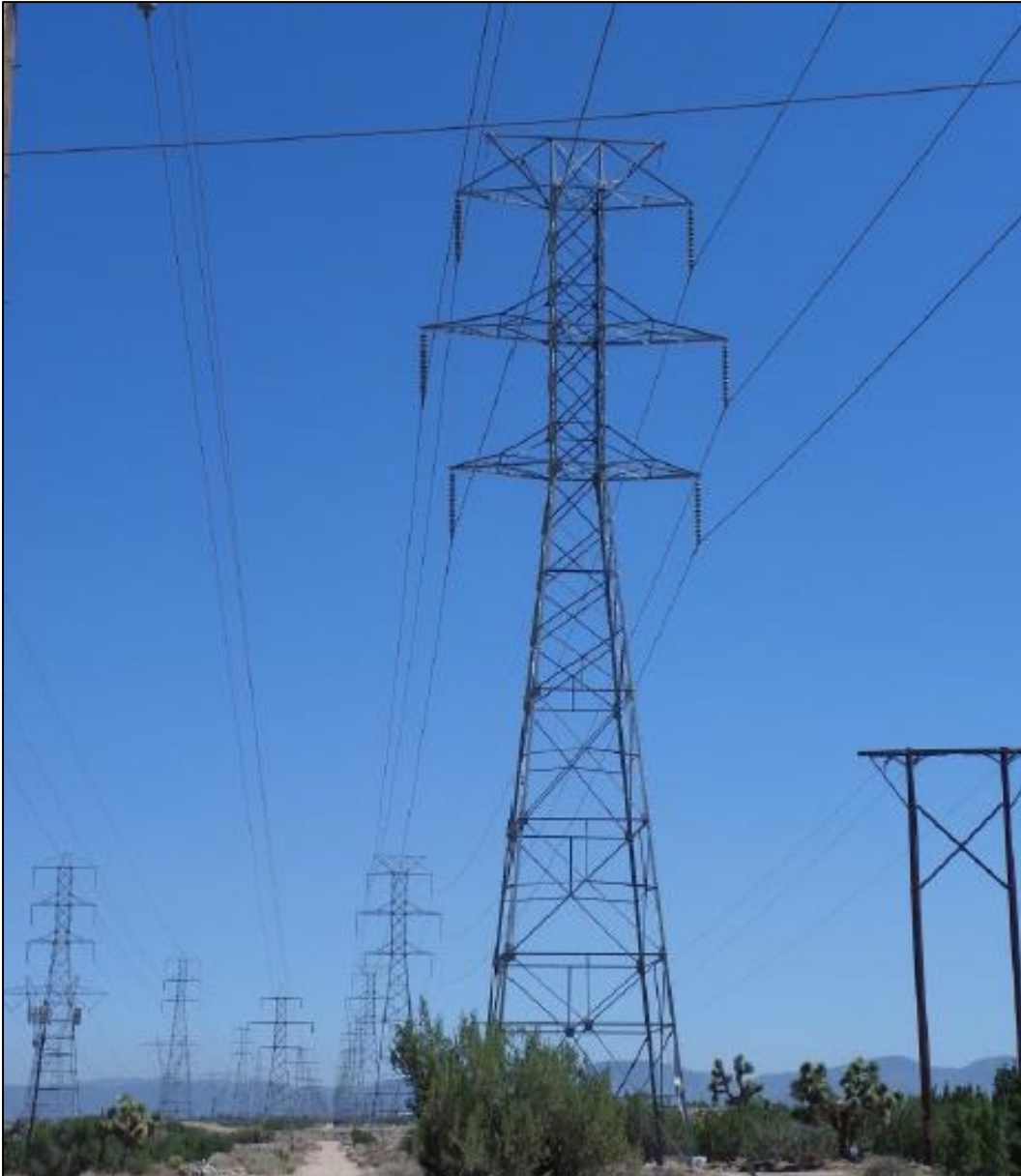
Figure 14: 132kV/275kV Powerline Double Circuit Suspension Towers
