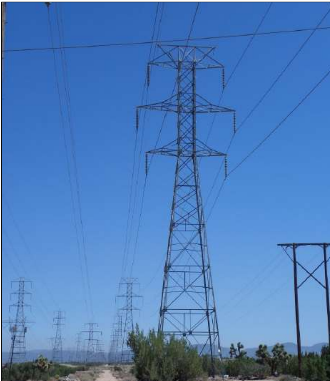
Figure 13: 132kV/275kV Powerline Double Circuit Suspension Towers
