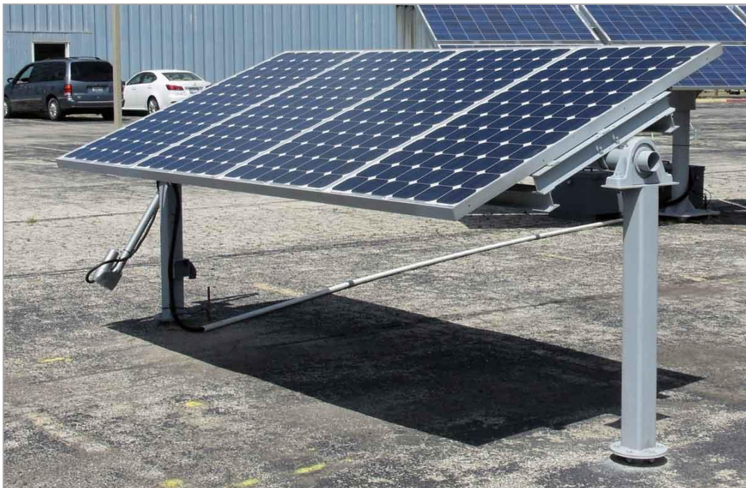
Figure 12 Example of PV Module mounted on Single Axis Tracker
