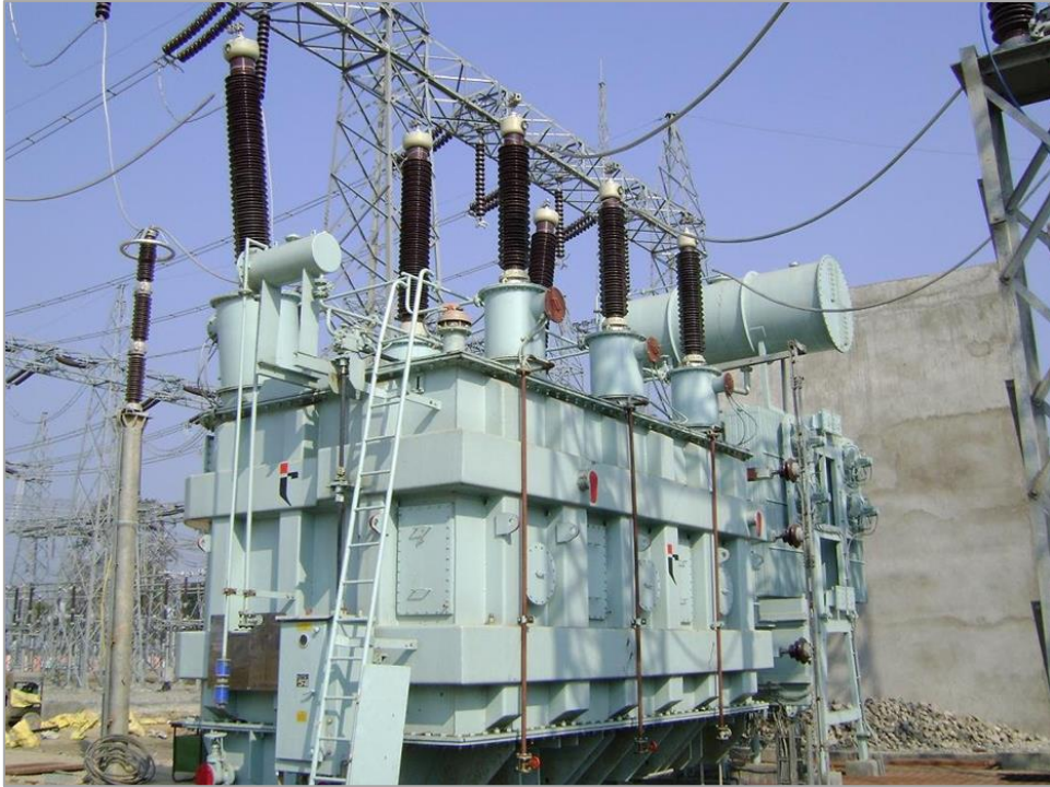
Figure 13: Example of Medium Voltage Transformer
