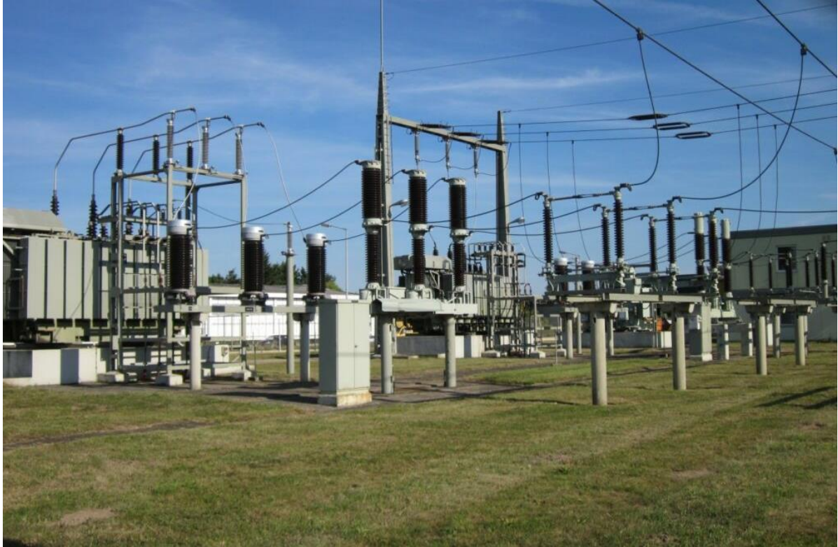
Figure 14: Example of High Voltage Substation (source: https://www.protoenergy.com/ )
