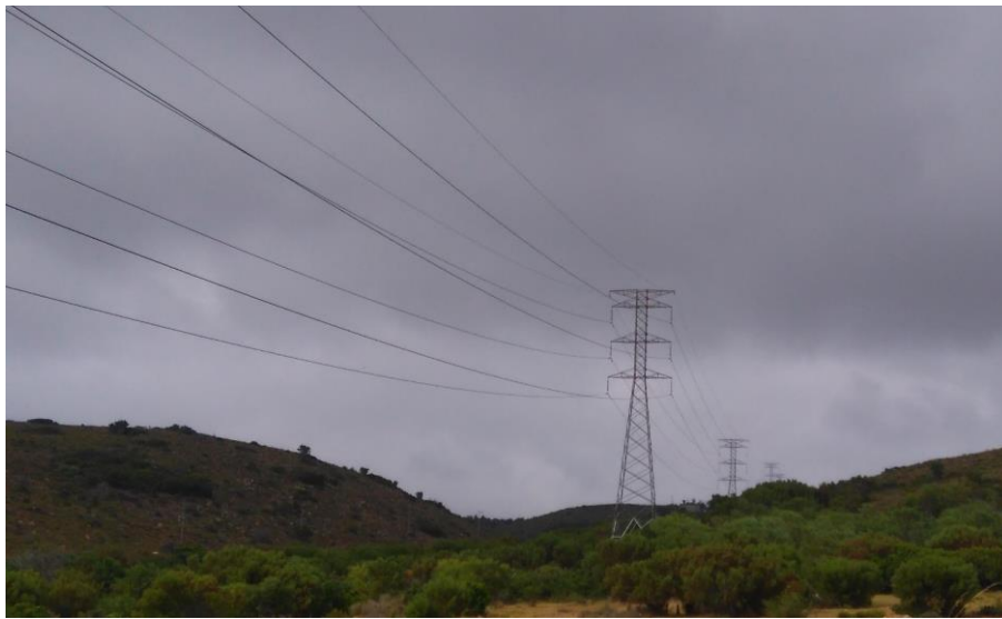
Figure 19: Example of a 132 kV transmission line
