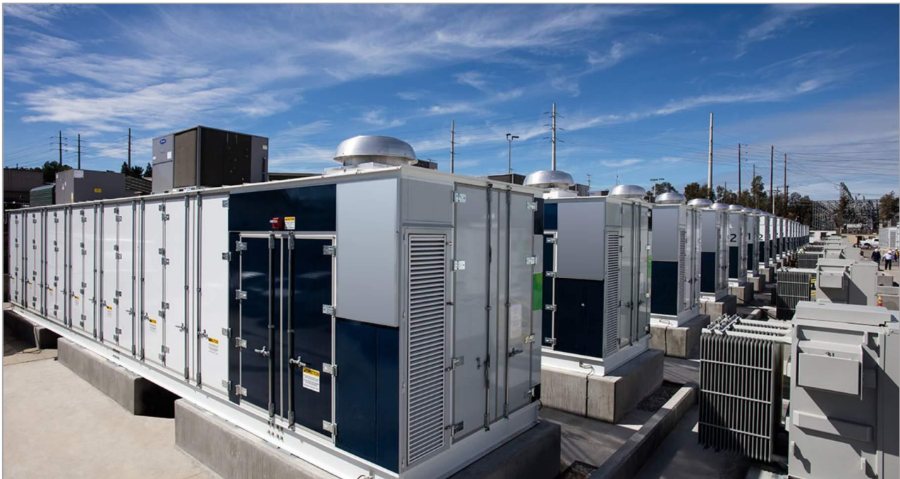
Figure 18: Example of BESS installation ( https://biiworld.com/ )
