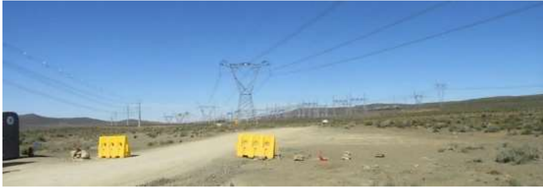
Figure 6-52: Eskom's Komsberg substation, viewed from the entrance along the Komsberg Road
