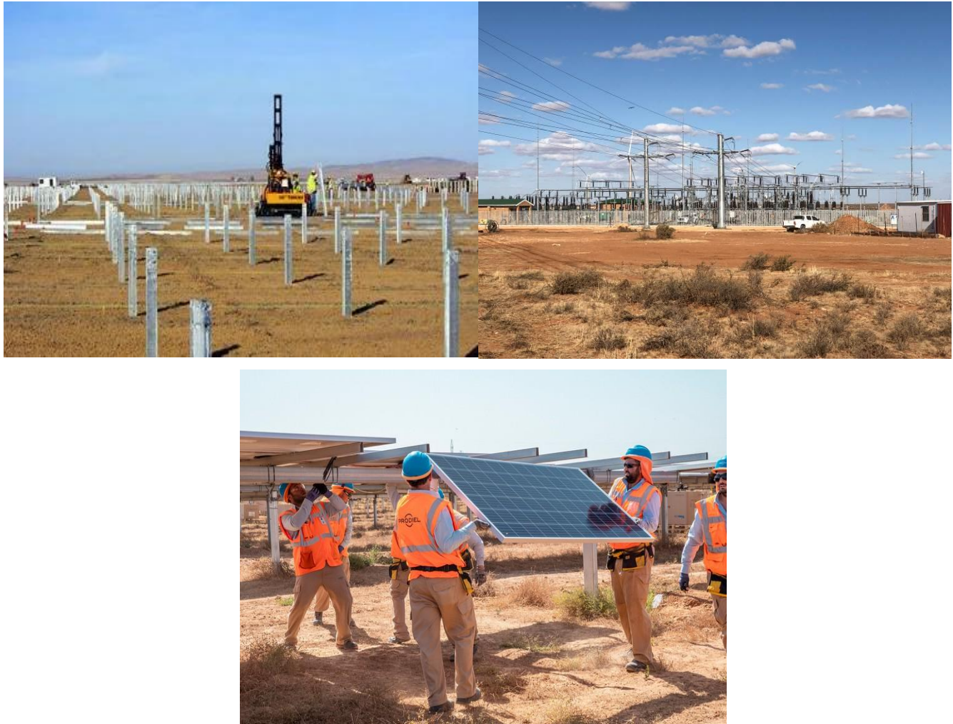
Figure 2-6: Photographs depicting the construction phase of a solar farm similar to Red Sands Solar East SEF. Source: www.power-technology.com , renewablesnow.com
