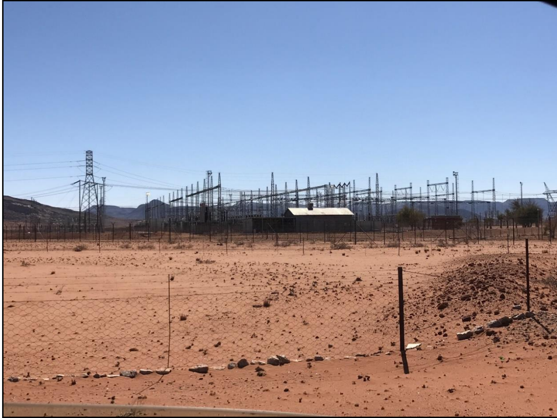
Figure 6-42: The Aggeneis Substation as seen from the N14
