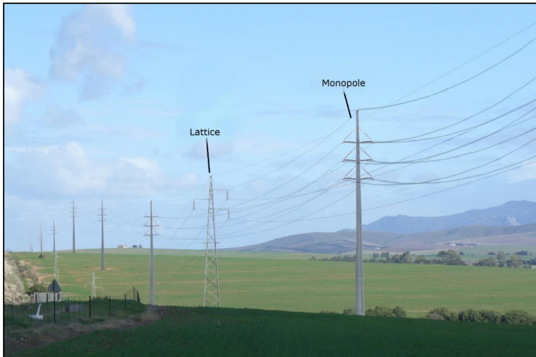
Figure 6-47: Examples of 132kV overhead power lines.
