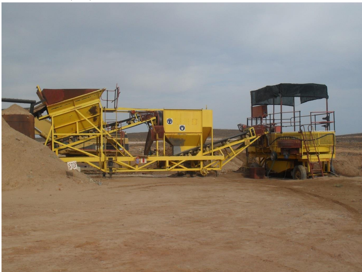
Photo 1: Mobile pan plant to be used
